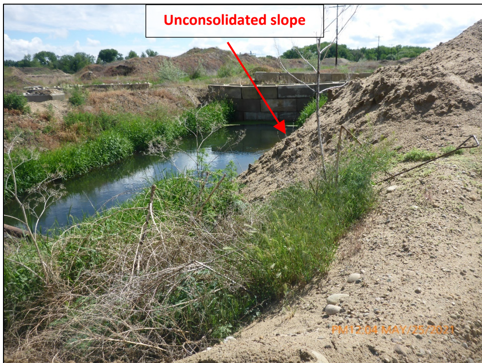
Photograph 22. View of unconsolidated and unstabilized sand and soil slopes immediately adjacent to the tributary of Center Point Canal.
