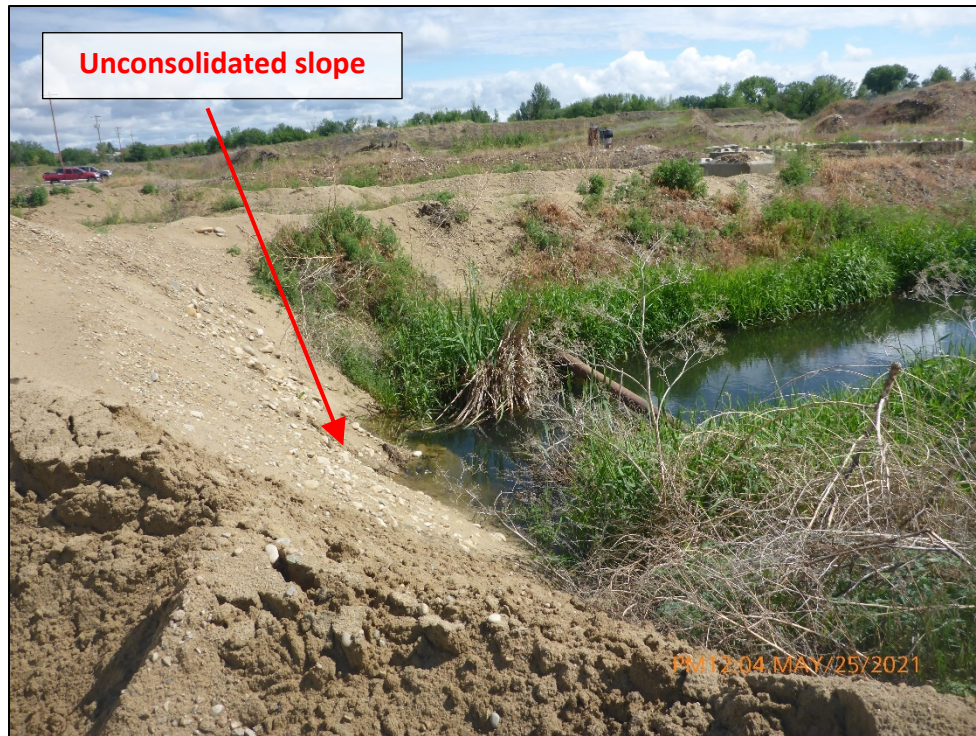
Photograph 23. View of an unconsolidated and unstabilized sand and soil slopes immediately adjacent to the tributary of Center Point Canal.
