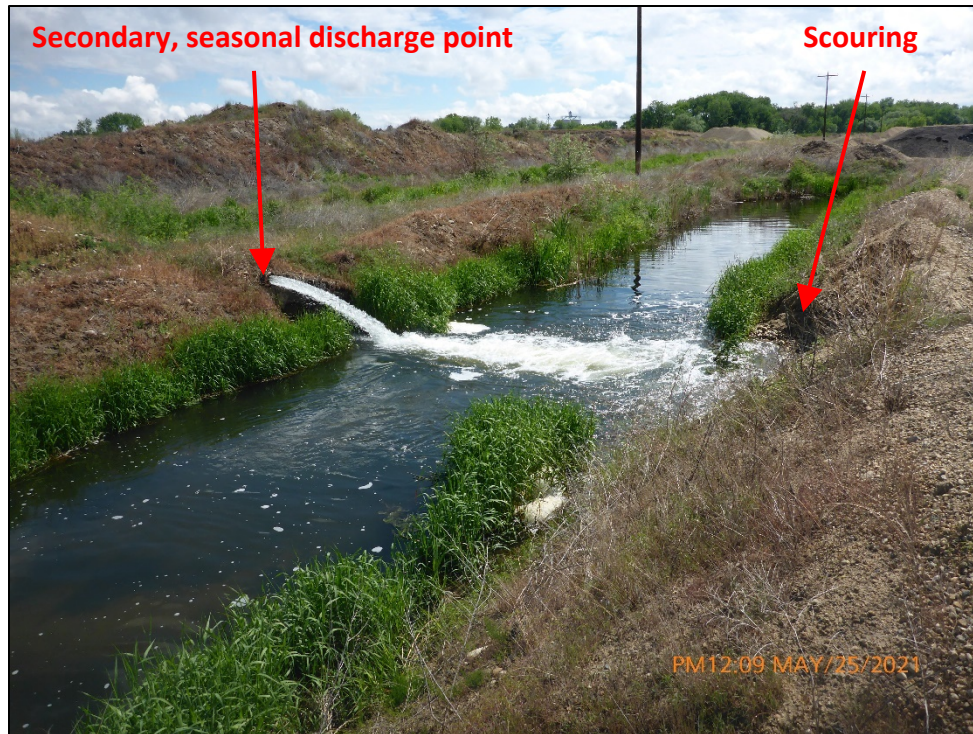
Photograph 15. Additional view, facing northeast, of the Facility's secondary, seasonal discharge point shown in Photograph 14. Note the scouring on the embankment of the ditch adjacent to the discharge pipe.
