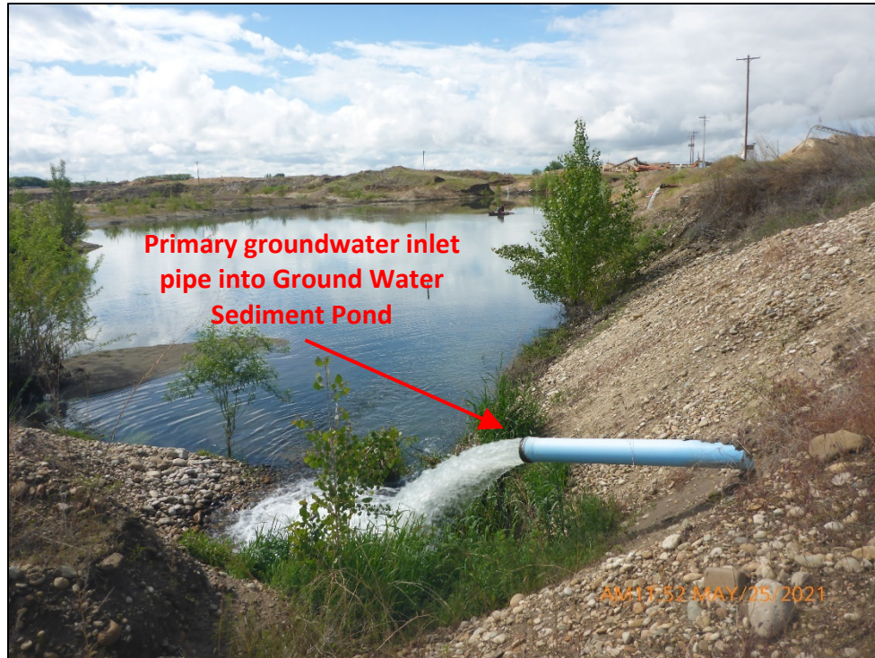
Photograph 7. View of the primary (year-round) inlet pipe that conveys groundwater into the Ground Water Sediment Pond.
