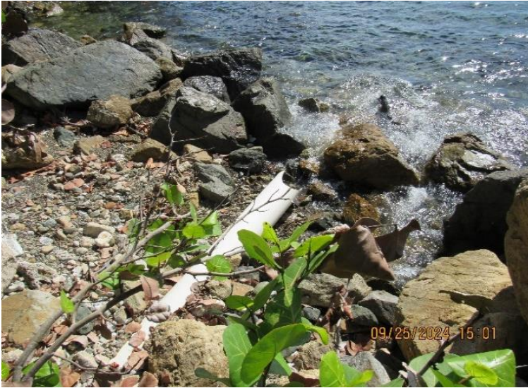
IMG 1402-Outfall 002. A 6-inch PVC pipe conveys stormwater runoff from uphill areas of Facility operations, including the LUB and BHA activities of the Facility. Discharges directly into Pacquereau bay.
