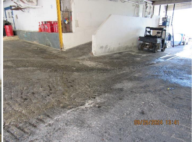
IMG 1384 -Stormwater flow path down gradient drain into a stormwater catch basin that discharges into Outfall 002.
