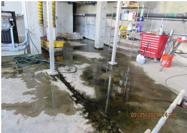
IMG 1392 -Evidence of algal growth in water that appears to be sipping through a concrete wall and ponds on the lower paved floor of the WWTP. The water is pumped from a sump basin into nearby Pacquereau Bay.
