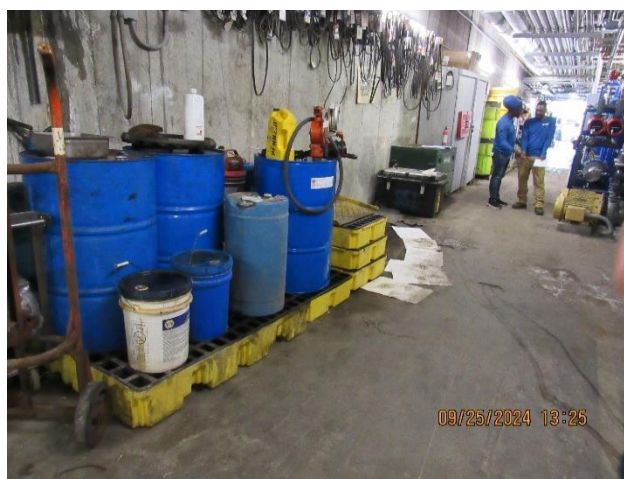
IMG 1369 -Plant Operation Area of Facility, where dispensing of lubricants, chemicals, and storage of used oil are carried out. Evidence that materials spills had recently occurred in the area.
