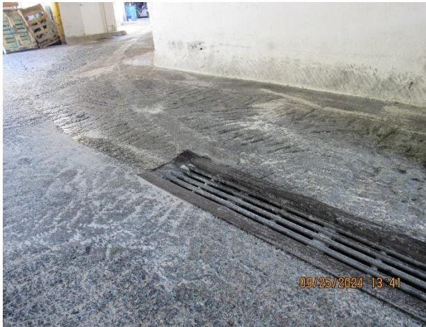
IMG 1386 -Evidence of dry-weather flow from BOH transporting oil-saturated sand into the stormwater catch basin, which drains into Outfall 002.
