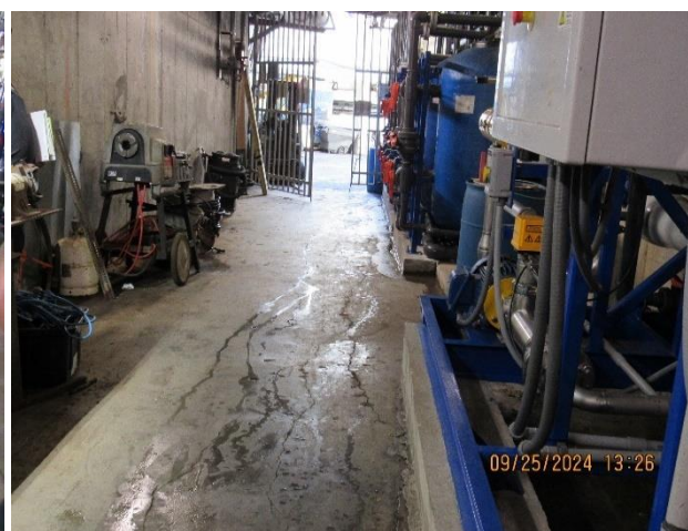
IMG 1371 -Facility's Reverse Osmosis Plant (ROP) in the Plant Operations Area. The inclined paved floor allows drainage of spillages out of the section into an area exposed to stormwater runoff flow.
