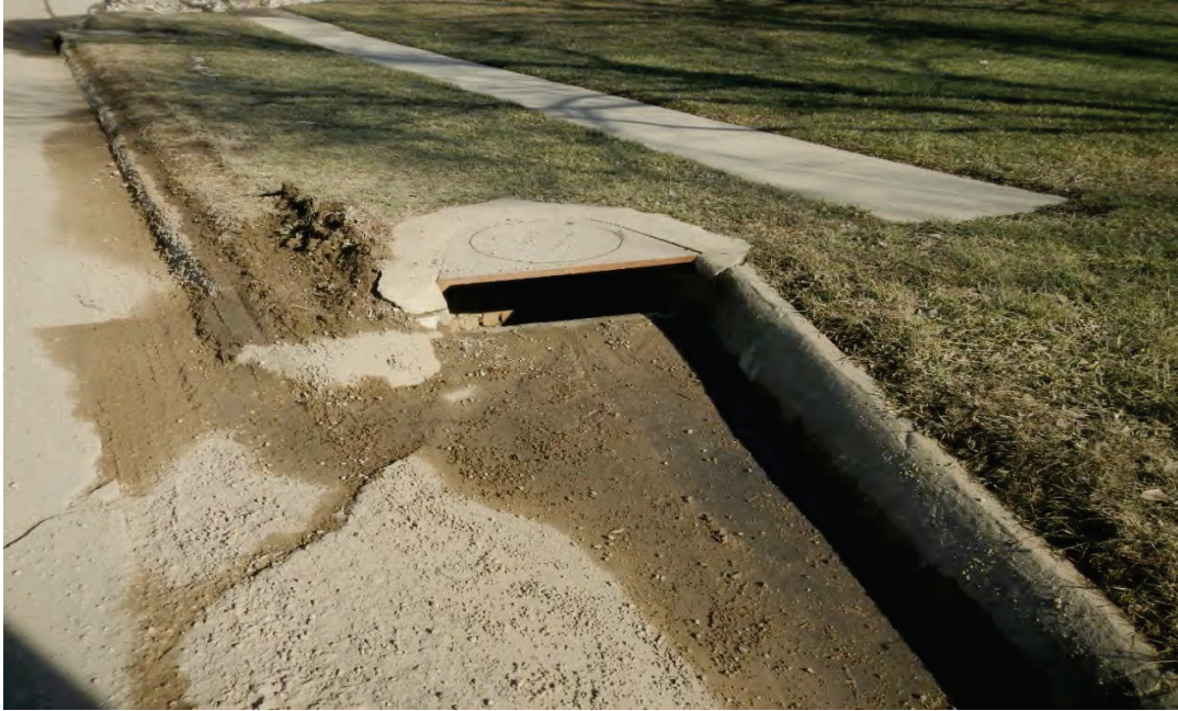
Photo 2, Sediment entering street stormwater inlet which is part of the MS4.
