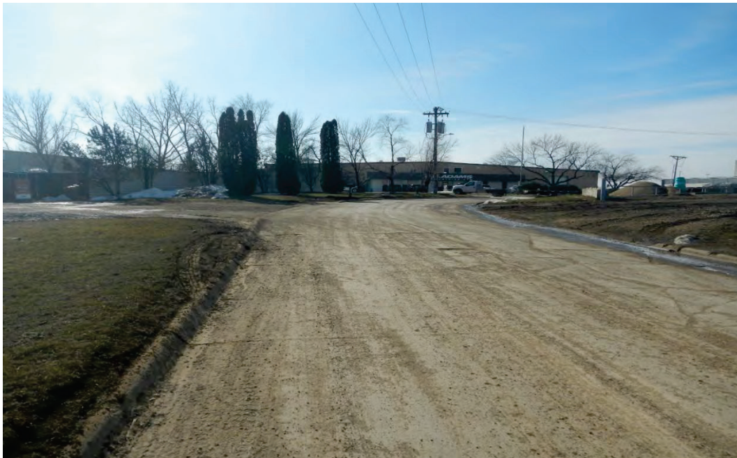
Photo 3, Sediment deposits at 11 th Street SW caused by vehicular activity.
