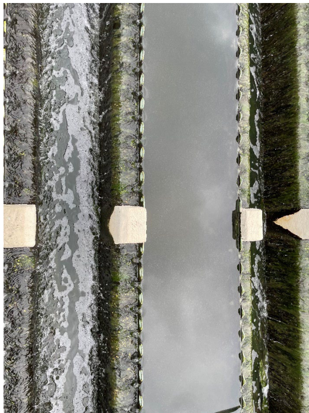
Photo #4. Pin floc was observed overflowing the weirs from the Final Sedimentation Tanks.
