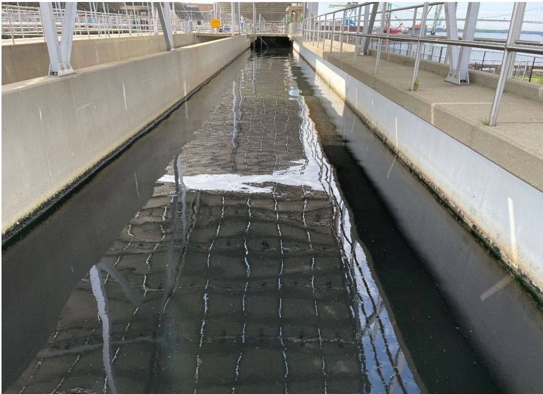
Photo #6. Fine bubbles were observed raising to the surface in the chlorine contact channel.
