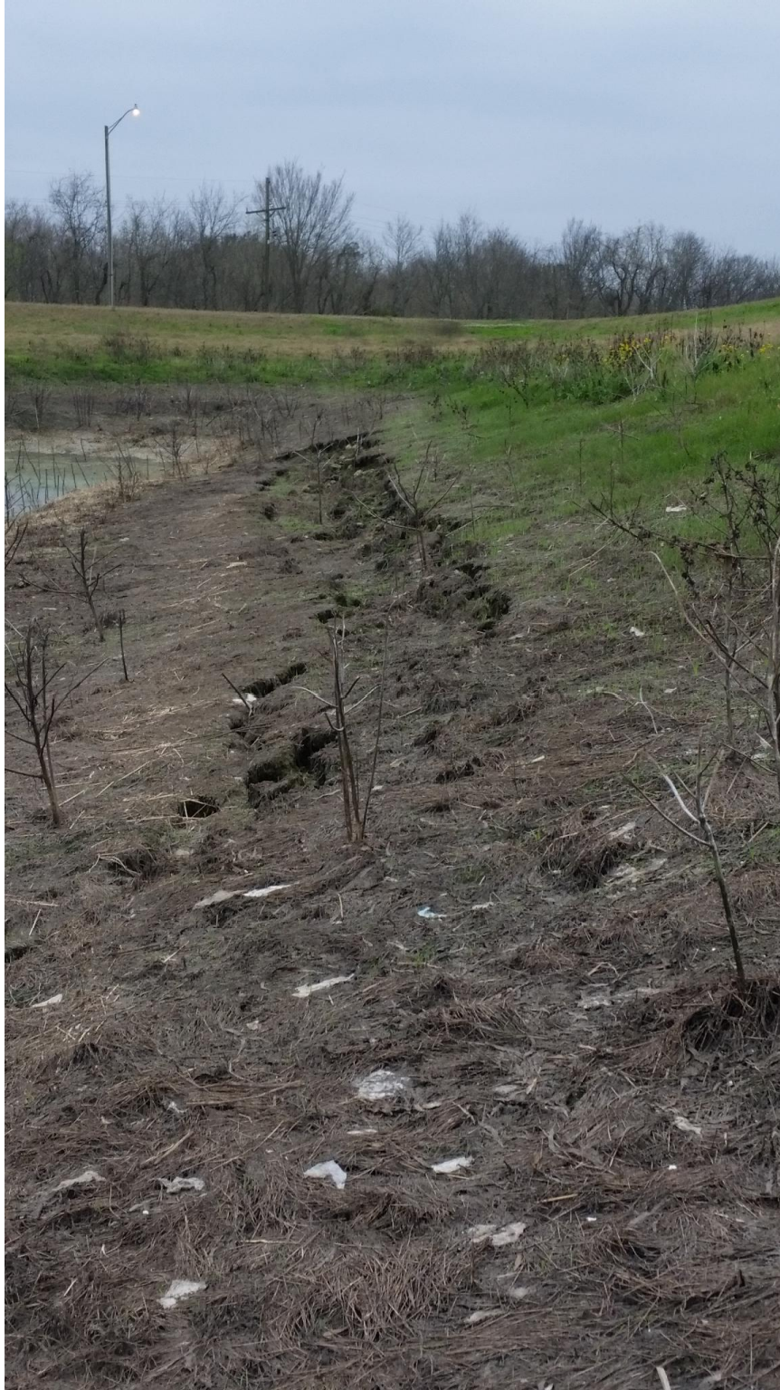
PHOTOGRAPH 5 – Slope Failure South Levee Looking East
