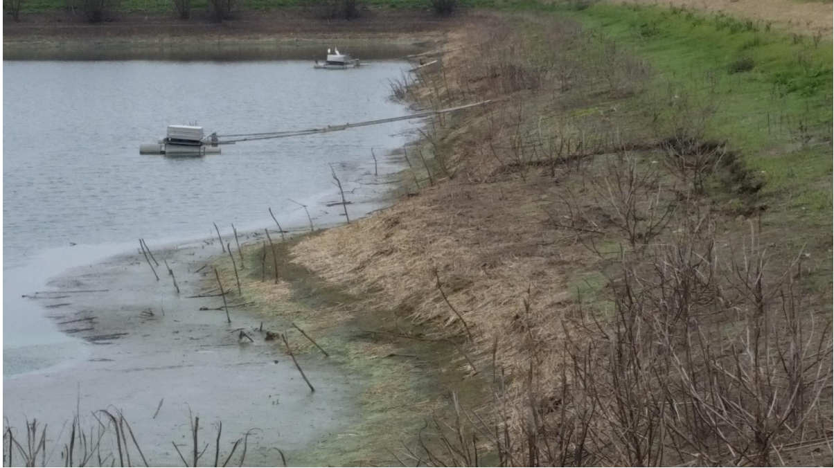
PHOTOGRAPH 2 – Slope Failure South Levee Looking East
