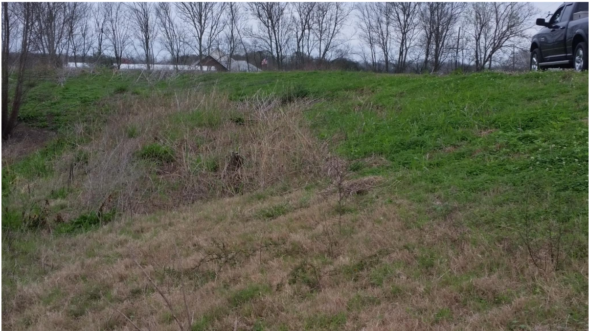
PHOTOGRAPH 3 – Slope Failure East Levee Looking North
