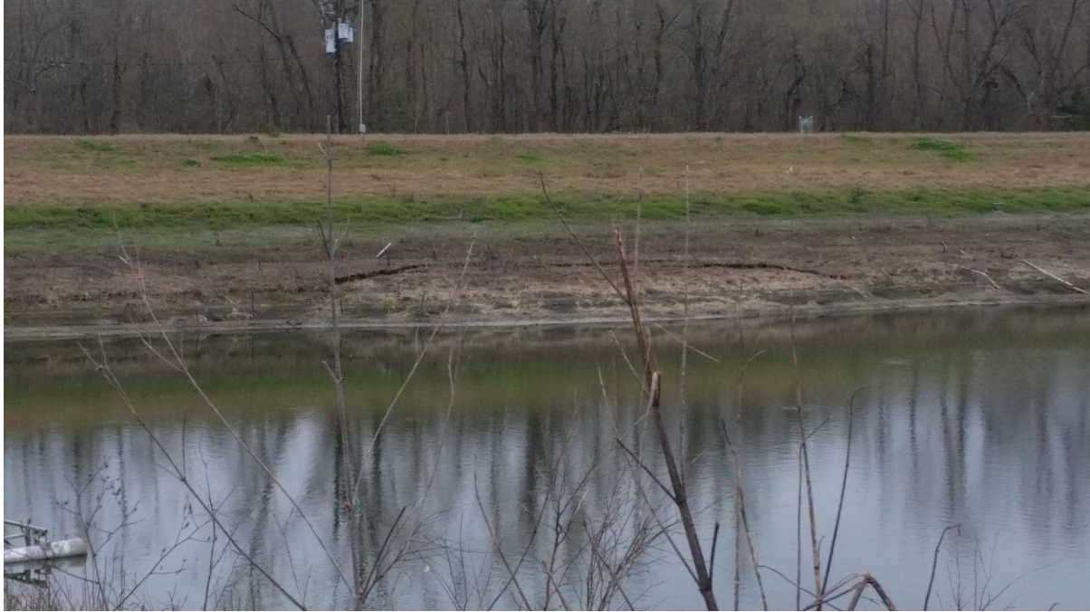
PHOTOGRAPH 4 – Slope Failure East Levee Looking East
