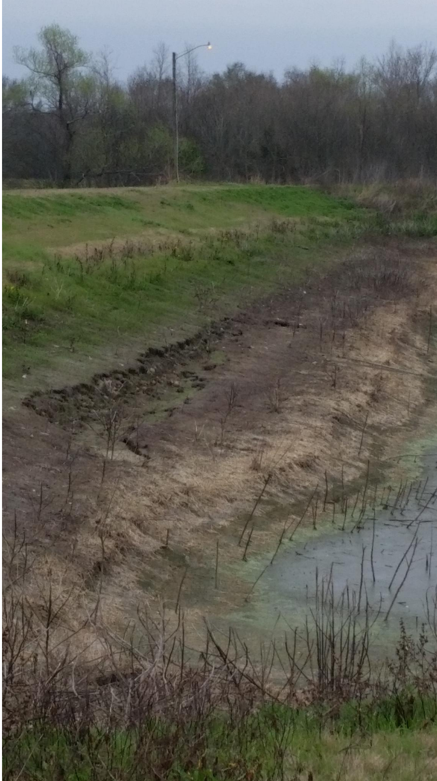
PHOTOGRAPH 1 – Slope Failure South Levee Looking West
