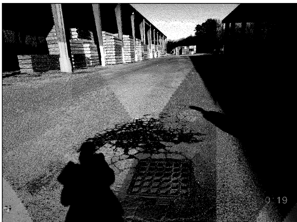
Photograph 20. View, facing north, of the northern catch basin in the mid-north area of the Facility. The catch basin is connected to the northwest detention basin
