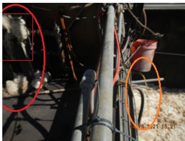
Photo 16. Post-aeration Basin. Sampling box indicated by the red boxed outline. Orange outline shows defoaming agent inflow. Significant foaming observed at the sampling box, indicated by red oval outline.
