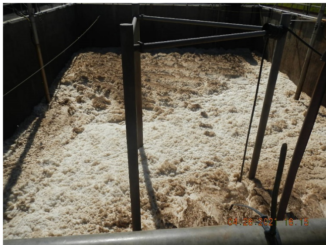
Photo 13. Post-aeration Basin interior holding tank.
