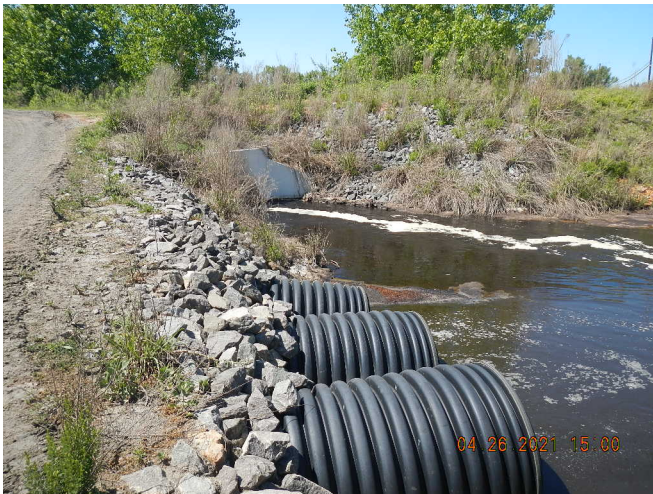
Photo 7. EQ Basin and EQ Basin Bypass Pipe outlets to the Inlet Ditch.
