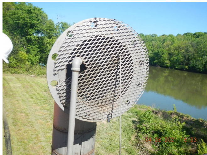
Photo 18. Defoaming agent discharge pipe, discharging into the Post-aeration Basin outlet to Outfall 001.
