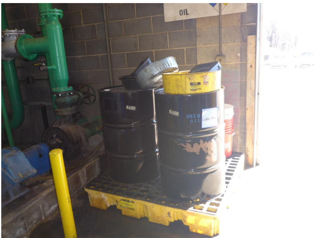
Photo 20: Three 55-gallon drums of used oil on a portable secondary containment pallet in the Chiller Room.
