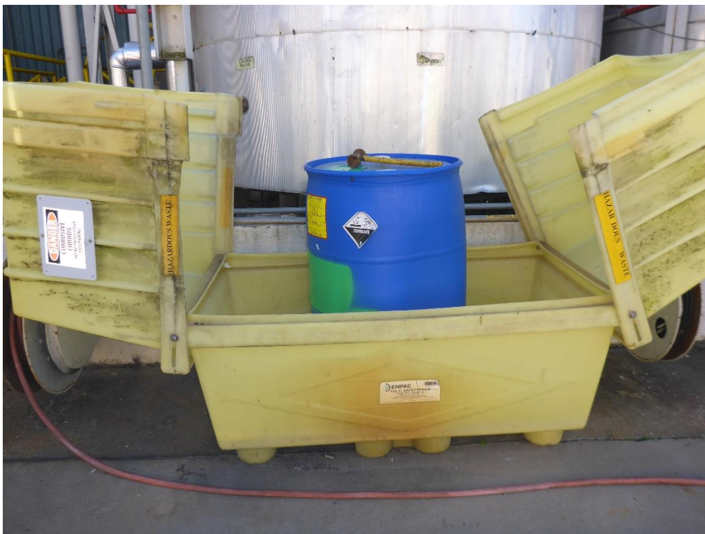
Photo 7: One 55-gallon drum inside a locked, plastic clam-shell secondary containment unit at SAA #6, which is used to accumulate hazardous waste MEA waste that is generated by sampling the MEA process. The clam-shell was labeled as SAA #6 and “danger corrosive liquids.” The drum was labeled hazardous waste MEA waste and identified with a corrosive DOT hazard placard.
