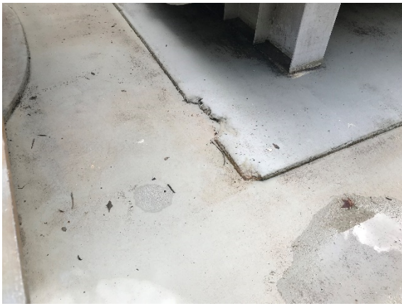
Picture 13: The base of the 10,000-gallon hazardous waste tank is chipped.
