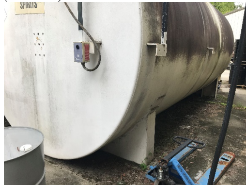
Picture 24: Double walled, 10,000-gallon Clean Solvent Tank
