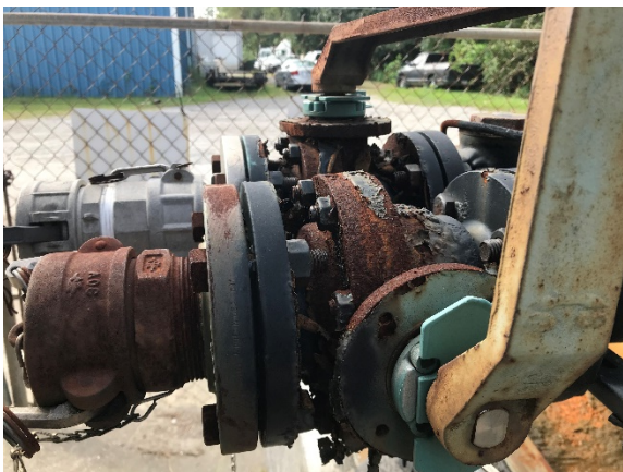
Picture 14: Sign of Rust and Paint Peeling in Ancillary Equipment associated with Hazardous Waste Tank #1
