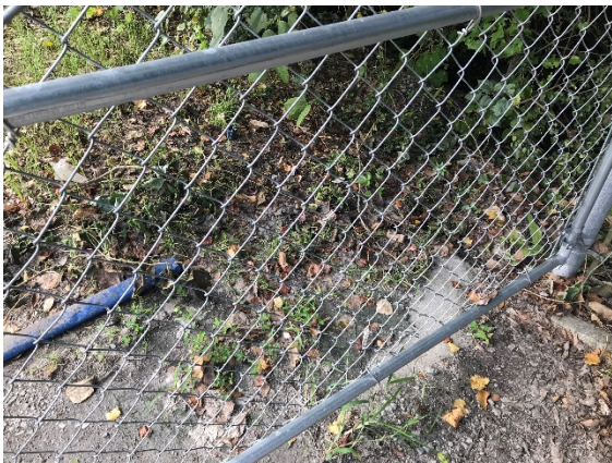
Picture 9: A pipe connected to a pump for discharging storm water containing hazardous waste to an unnamed tributary of a creek
