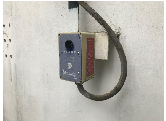
Picture 18: High Level Tank Alarm Switch was disconnected for Hazardous Waste Tank #1
