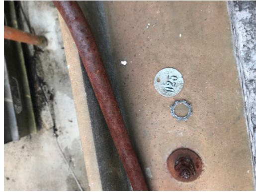
Picture 22: Tags associated with the Ancillary Equipment observed in the ground and rusted ancillary piping associated (Tank #1)
