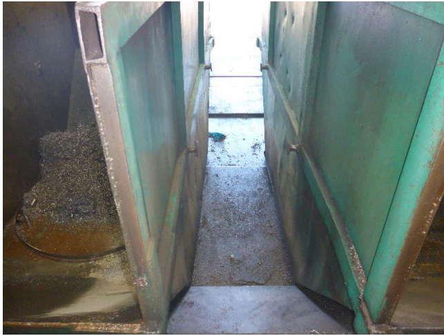
Photo 16: The top of the 2,500-gallon metal fabricated storage tank located below the three large hoppers just off the edge of the loading dock at the Chip Dock.
