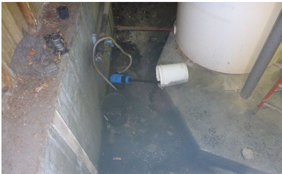
Photo 12: Dirty liquids observed on the floor surrounding the concrete pad beneath the 2,000-gallon vertical storage tank.
