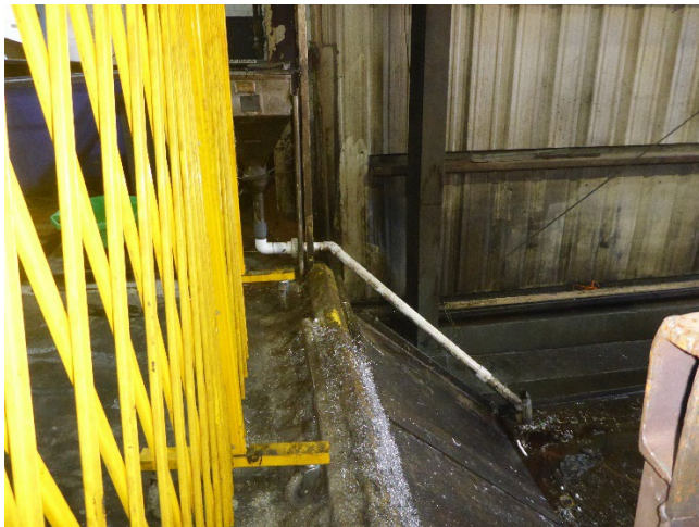
Photo 17: Funnel that is connected through PVC piping into the 2,500-gallon metal fabricated storage tank beneath the three large hoppers at the Chip Dock.
