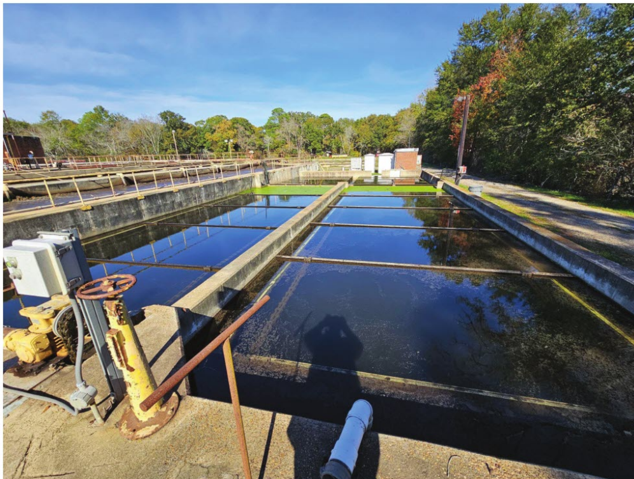
Primary Clarifiers for Train #1
