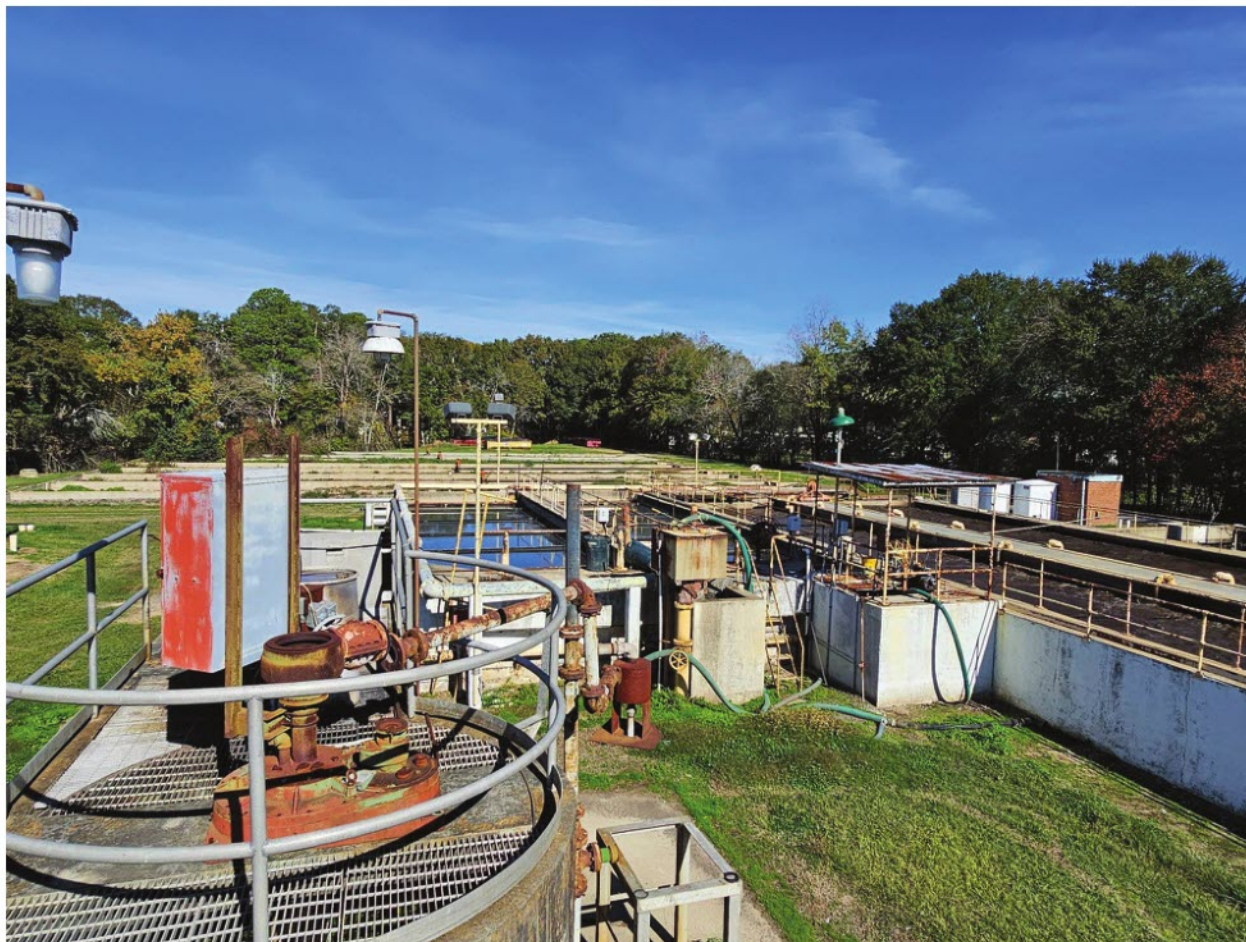
Aerial View of Train #1 with Dual aeration and Clarification
