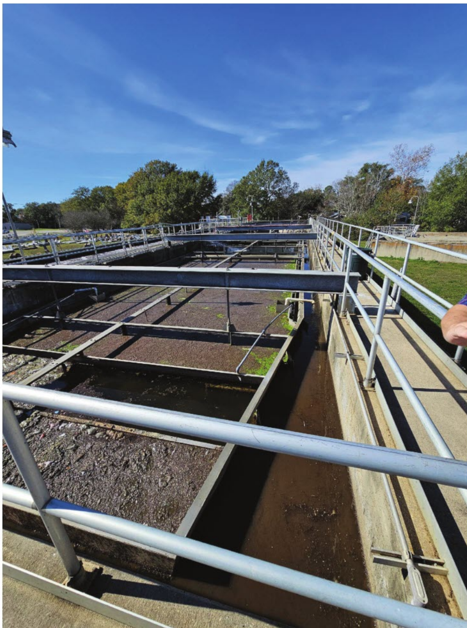
Boat Clarifier Train #2
