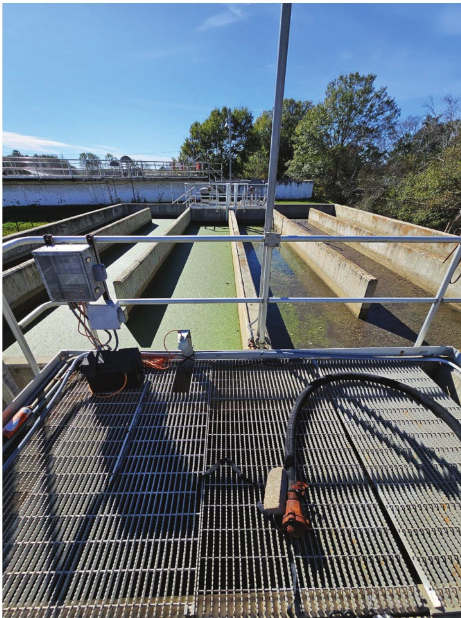
Chlorine Contact Chamber
