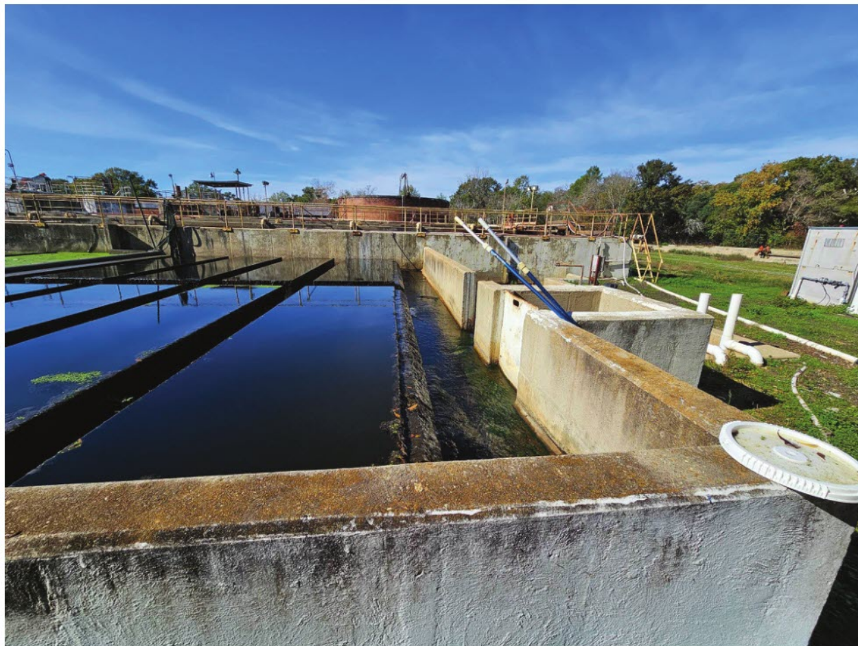
Secondary Clarifiers for Train #1 prior to disinfection
