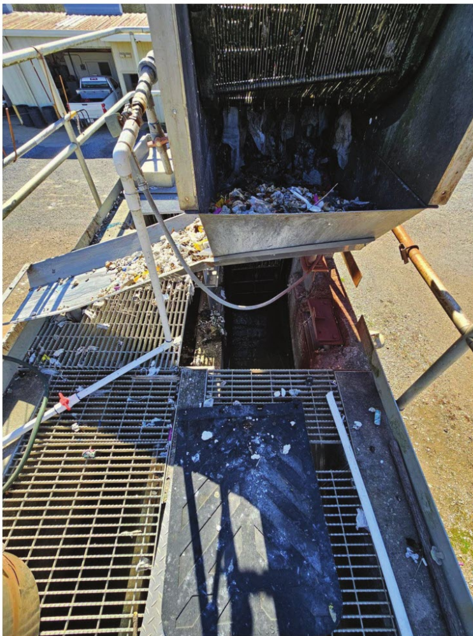
City of Eunice mechanical bar screen and grit chamber
