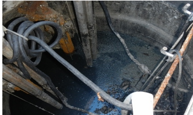
Photo 4. System Sump Pumps
