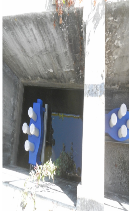
Photo 2. Chlorine and Dechlorination Tablet Tanks
