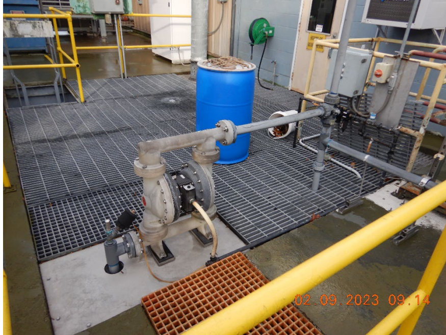
56: DSCN1183 Description: Pump near sump Location: Building 69 Area Camera Direction: Northwest Date/Time: 2/9/23, 9:14 a.m.
