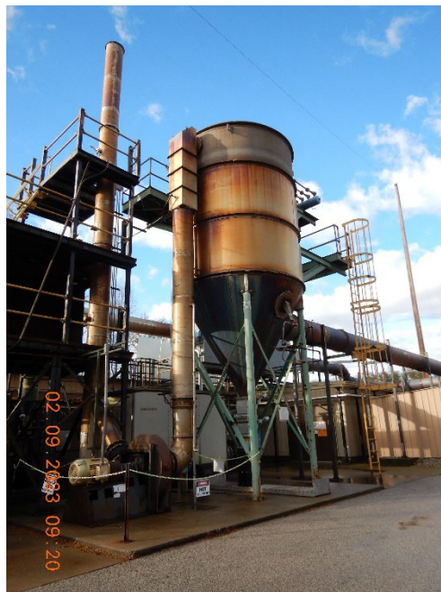
57: DSCN1184 Description: Dust collector for APE 1236 Location: Building 69 Area Camera Direction: Southwest Date/Time: 2/9/23, 9:20 a.m.
