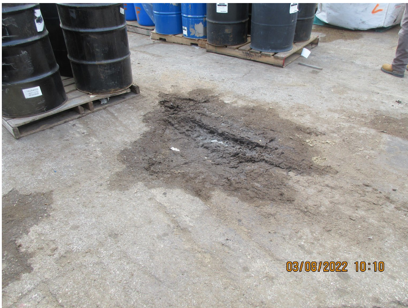
Photo 2 – Damage to Asphalt in Area of Row 14 of Unit 217
