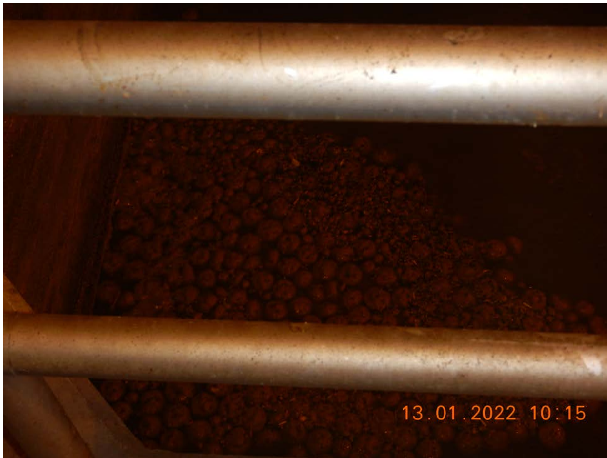
Photograph of the accumulated "grease balls" within the northside wet well. Note: these grease balls are removed by skimming the surface with a net. January 13, 2022. 10:15 AM (DSCN 2071). Photographed by D. Esparza.
