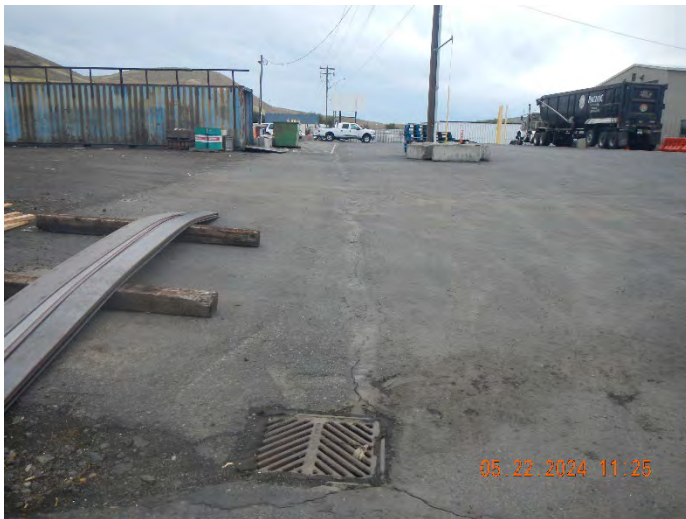
Photo #:07 (DSCN3746) Description: Facing east, photo of central catch basin identified as Outfall 001. Filter/sediment fabric installed within catch basin. Catch basin is located northeast of the New Steel Building.
