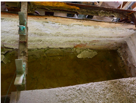
Photo #5 – Out of service zinc plating large barrel line tank.
