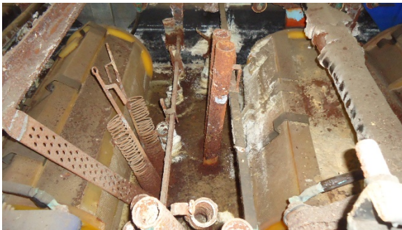
Photo #11 – Out of service zinc plating large barrel line tank.
