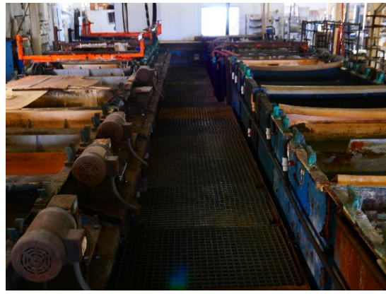
Photo #8 – Out of service zinc plating large barrel line tanks.
