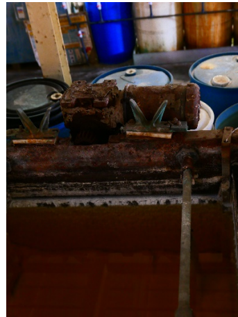
Photo #12 – Out of service zinc plating large barrel line tank.
