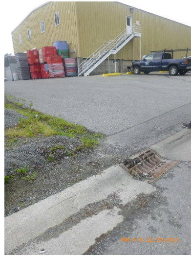
Photo #:22 (017) Description: Storm drain located in the southeast area of the site.
