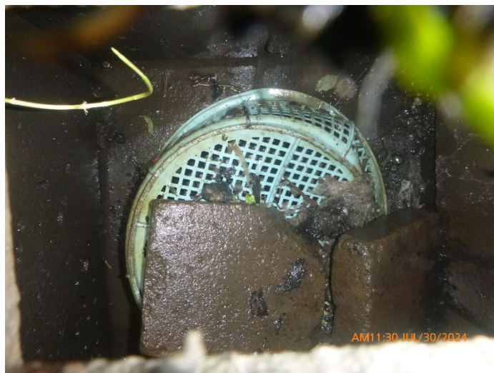
Photo #:18 (P1010220) Description: Northwest storm drain with blue bucket weighed down with a rock.
