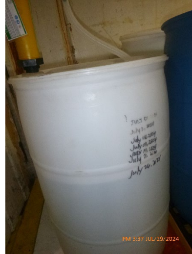
Photo #:10 (P1010201) Description: Sodium Hypochlorite storage.
