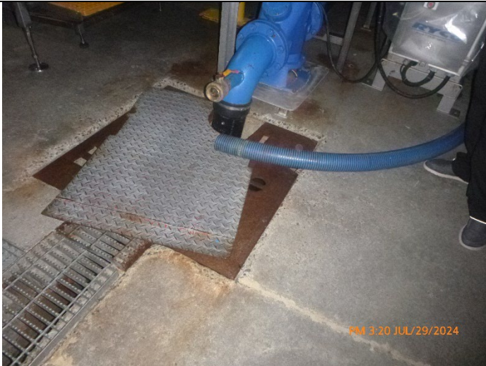
Photo #:27 (P1010185) Description: Main sump for processing waste before discharging to AWWU.
