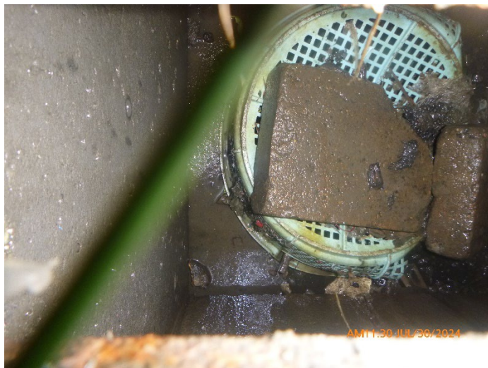
Photo #:19 (P1010121) Description: Northwest storm drain with blue bucket weighed down with a rock.
