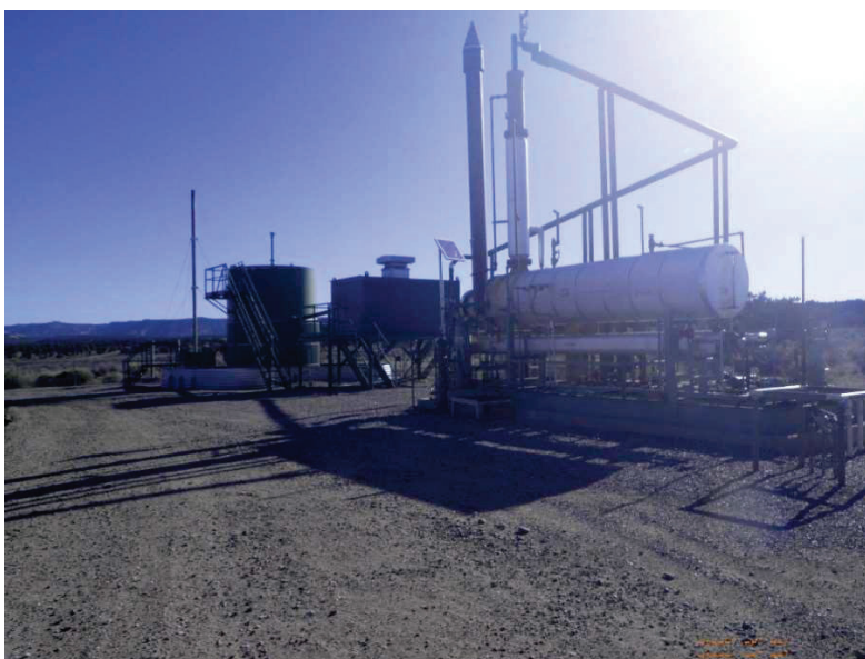
Figure 3: Ute dehydrator reboiler and tank no longer connected. RIMG0022.jpg
