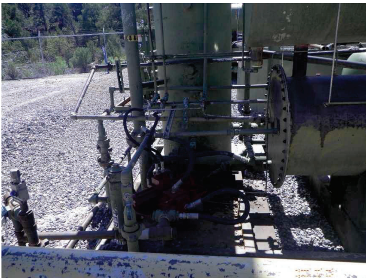
Image #9: Argenta Dehydrator #2 pump, RIMG0016.JPG.
