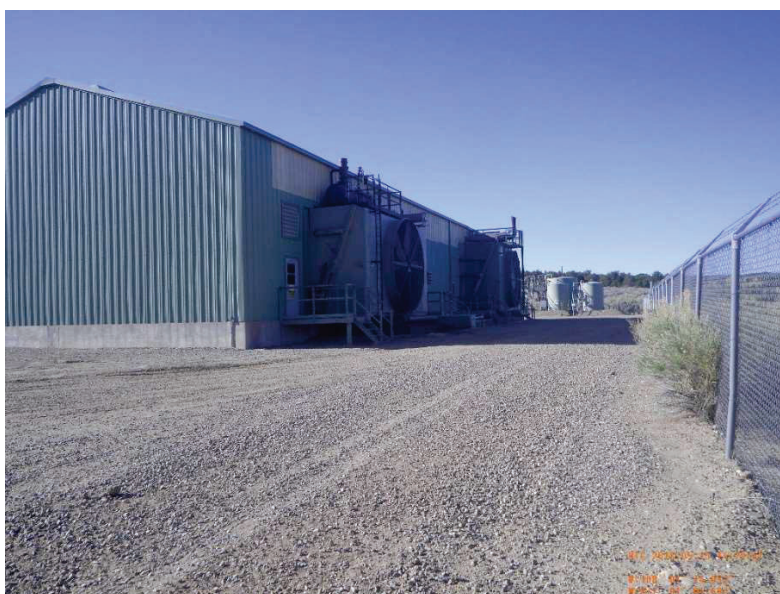
Image 4: Ute backside of engines, catalyst part of muffler, Engine #3 closest and Engine #1 farthest away. RIMG0023.jpg
