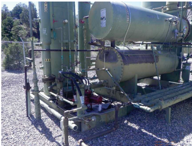
Image 8: Argenta Dehydrator #1 pump, RIMG0015.JPG
