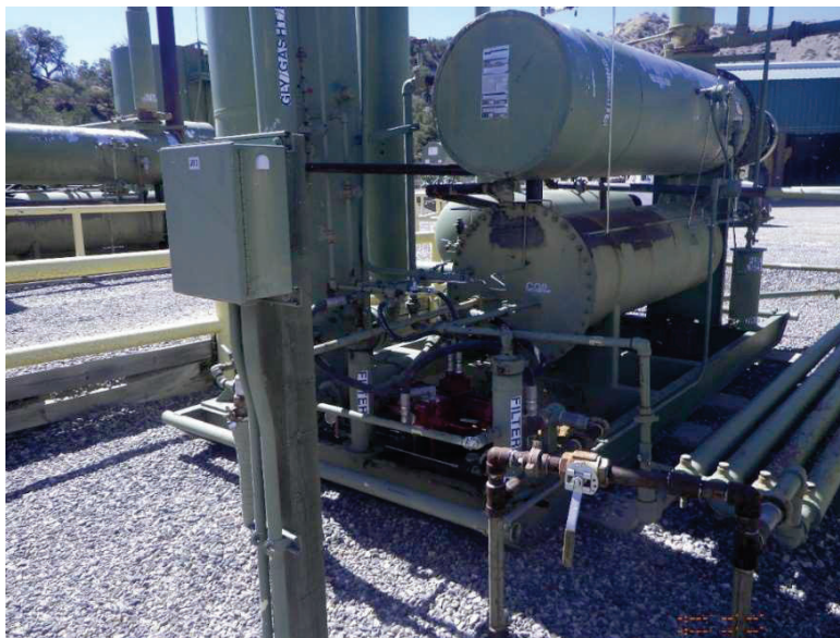
Image 12: Argenta Dehydrator #3 pump, RIMG0019.JPG
