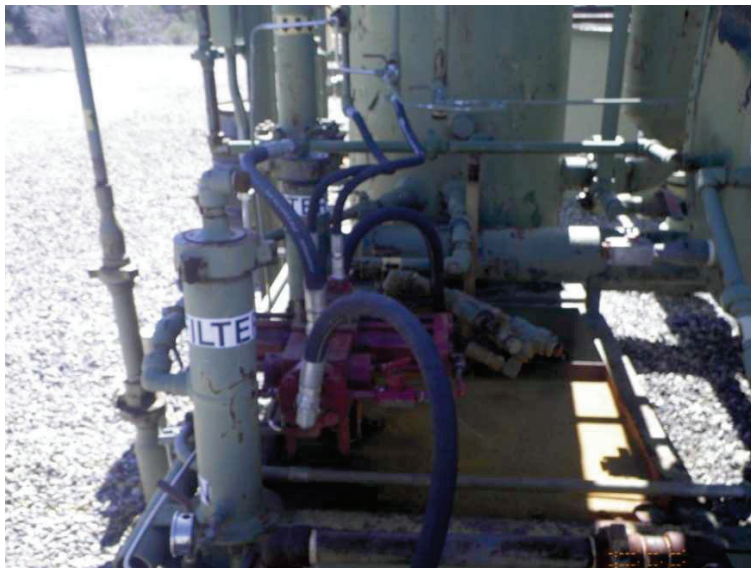
Image 13: Argenta Dehydrator #4 pump. RIMG0020.JPG
