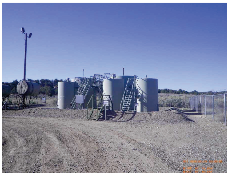
Image 5: Ute tanks. Two larger tanks are condensate in back, tank front right is used oil, middle tank is new oil and tank on left is antifreeze. RIMG0024.jpg
