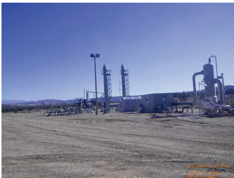
Image #8: Ute Inlet on right and two dehydrator contactors (not operating). RIMG0027.jpg
