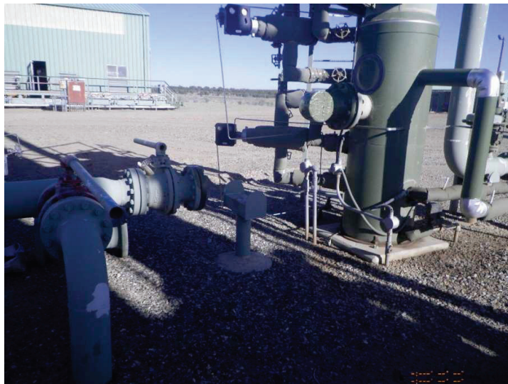
Figure 2. Ute showing the blinded off line of gas to the dehydrator. RIMG0021.jpg
