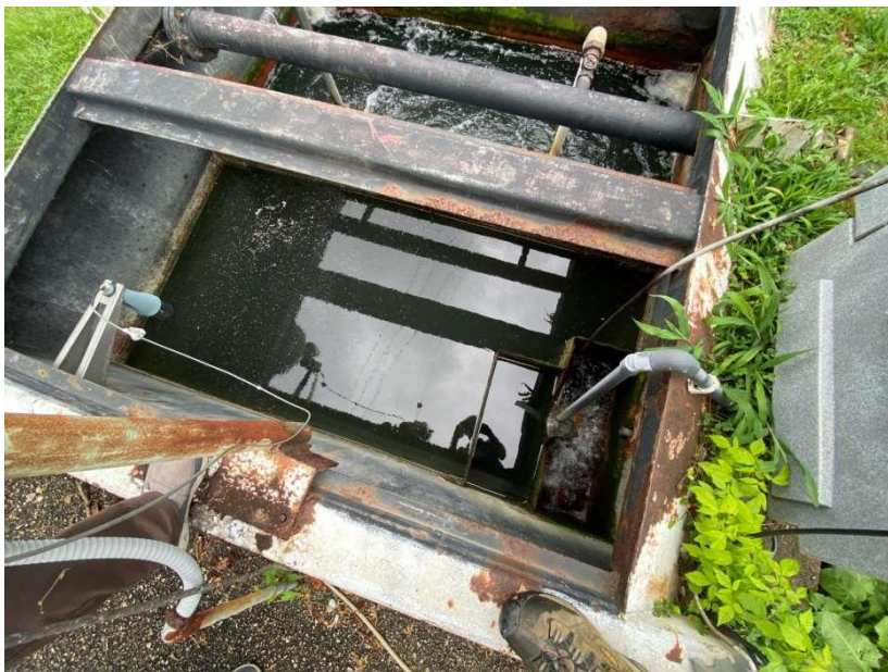
Figure 6: Photo of the chlorination chamber.
