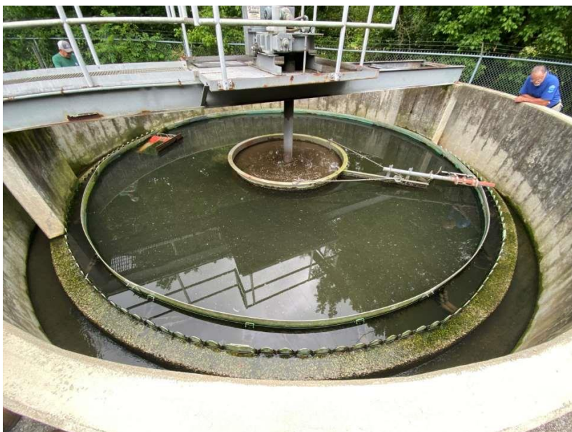
Figure 5: Photo of the final clarifier.
