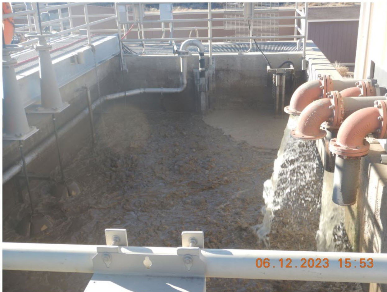
View of WWTP's pre-air basin. Bar screen and entrance headworks on right side of photograph. (DSCN2678). Photographed by D. Esparza
