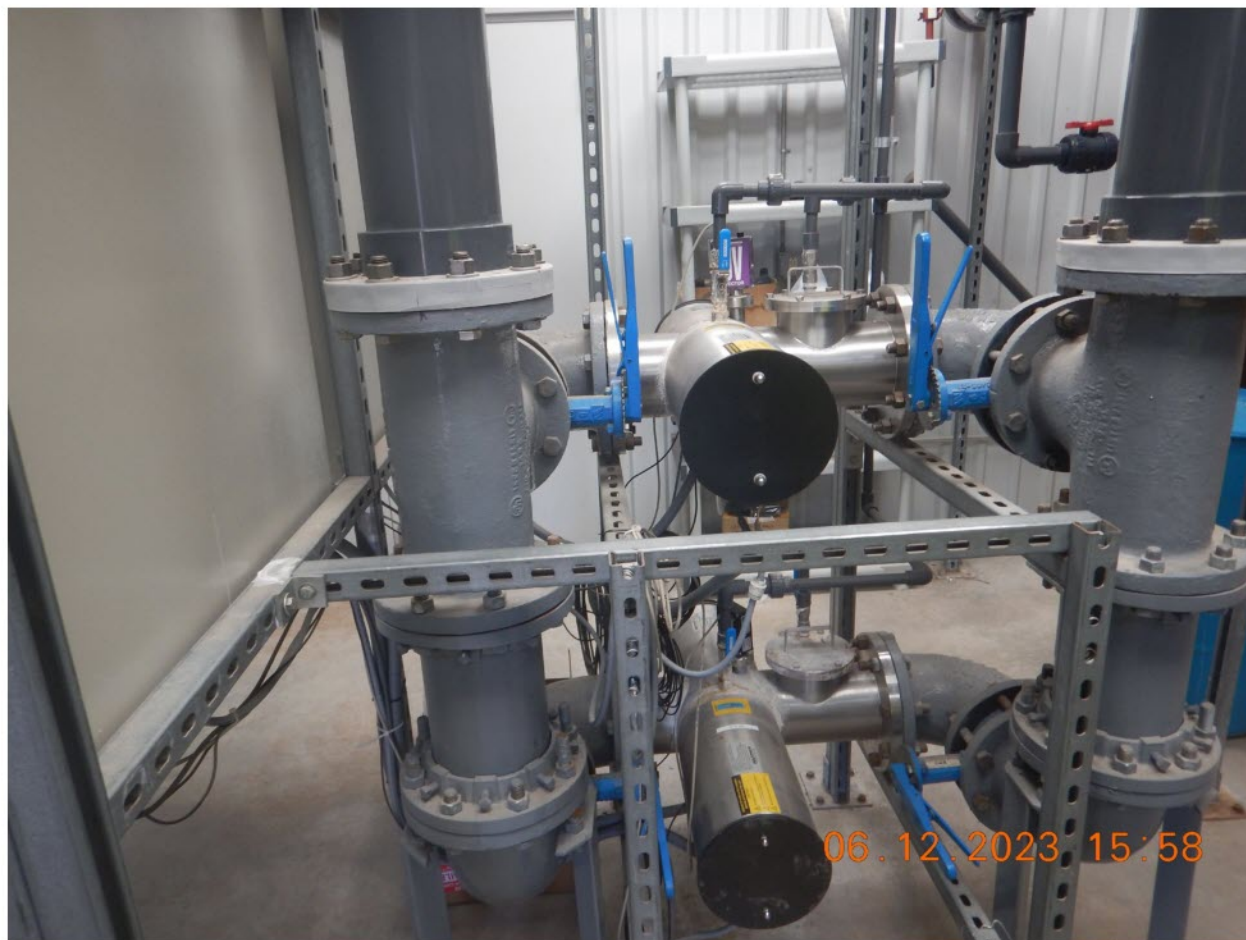
View of the ultraviolet (UV) disinfection treatment system. (DSCN2682). Photographed by D. Esparza
