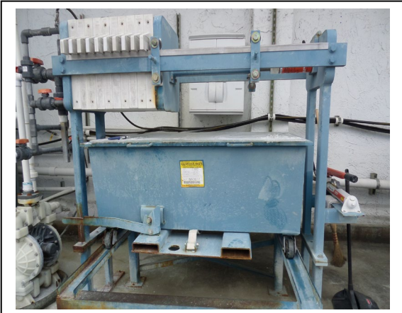
H & S. Wastewater Pretreatment System. H & S closed the hopper and marked it with an indication of the hazard. Photograph 9 taken at 12:23 p.m.
