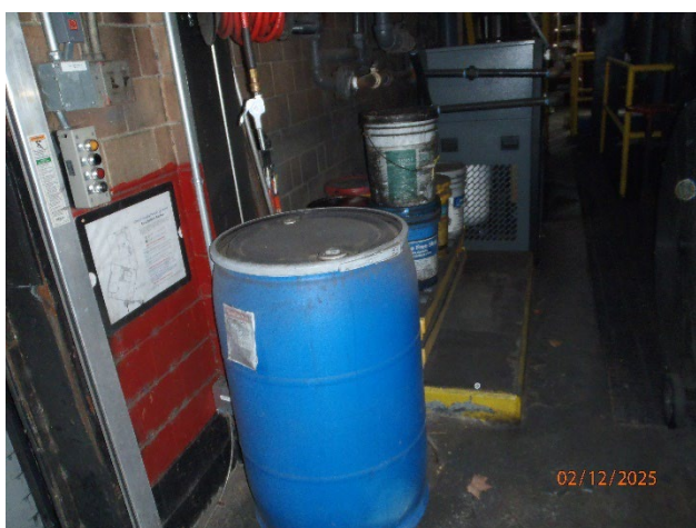
Picture 47 – Central Heating Plant UW aerosol cans
