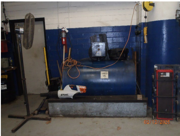
Picture 36 – Garage Used Oil Tank
