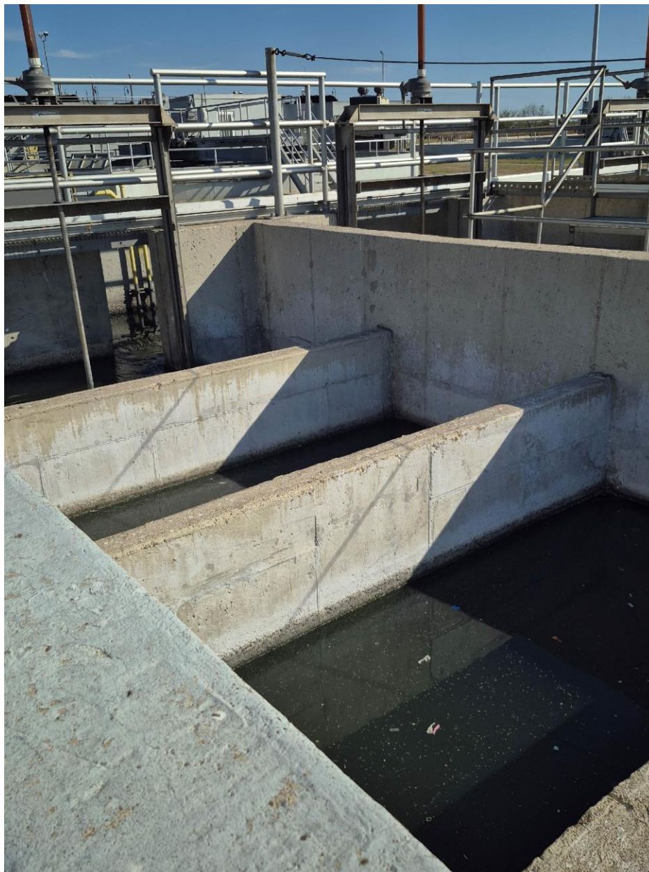
Chlorine Contact Chamber
