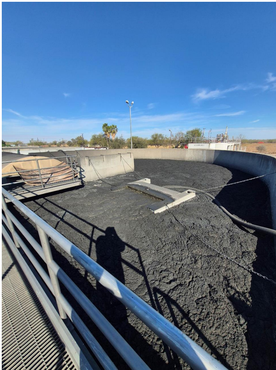
Aeration Basin with Non-Working Rotors
