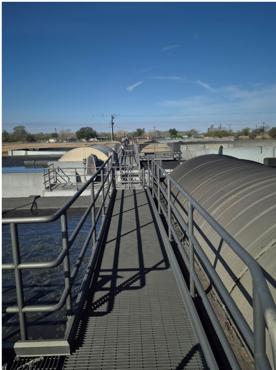
Working Aeration Rotors
