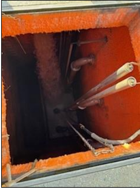
Photo 3. Davis Lane Lift Station (One of the three main lift stations discharging to the wastewater plant)
