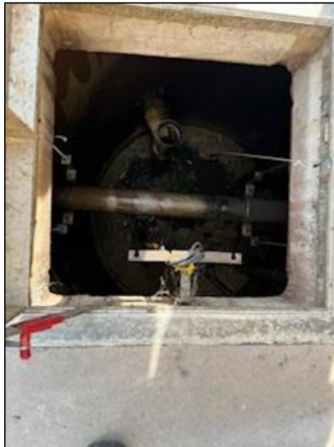
Photo 2. Stables Lift Station
