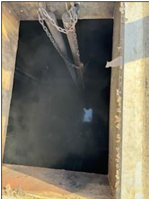
Photo 4. Kodak Lane lift station
