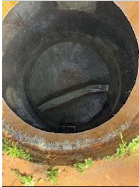
Photo 1. Manhole located at Stables Lift Station.
