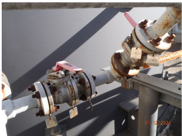
Picture 42 – U1-V613 Hazardous Waste Tank BB tags
