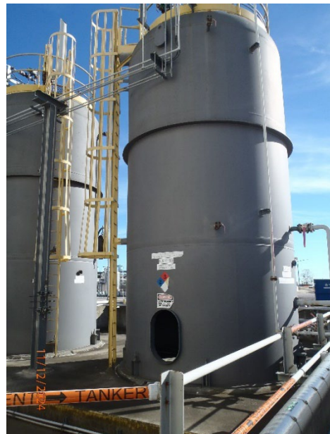
Picture 41 – U1-V613 Hazardous Waste Tanks
