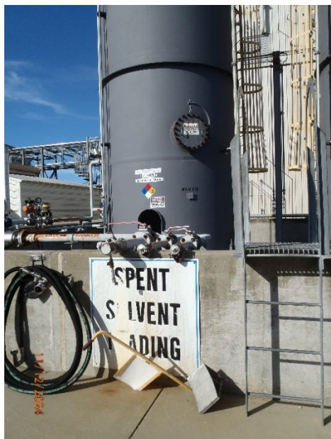
Picture 43 – U1-V613 Hazardous Waste Tank connection ports
