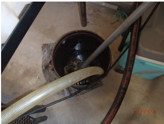
Picture 39 – E15 Building unlabeled and open Used Oil container
