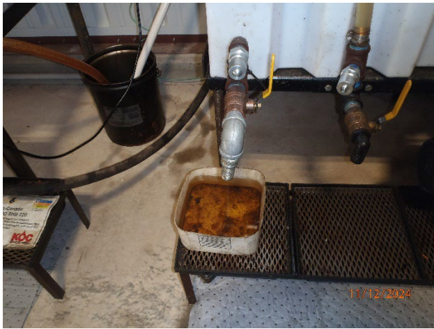
Picture 37 – E15 Building unlabeled and open Used Oil container
