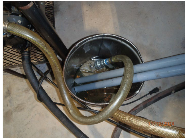
Picture 36 – E15 Building unlabeled and open Used Oil container
