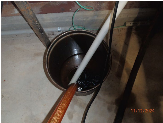
Picture 38 – E15 Building unlabeled and open Used Oil container
