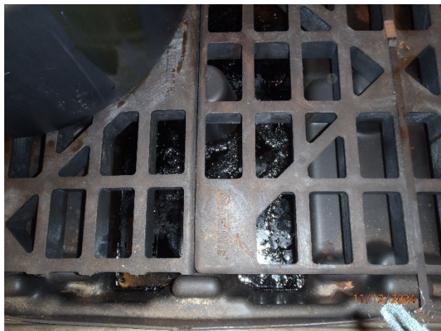
Picture 21 – TFE N1 Plant SAA secondary containment needs cleanout
