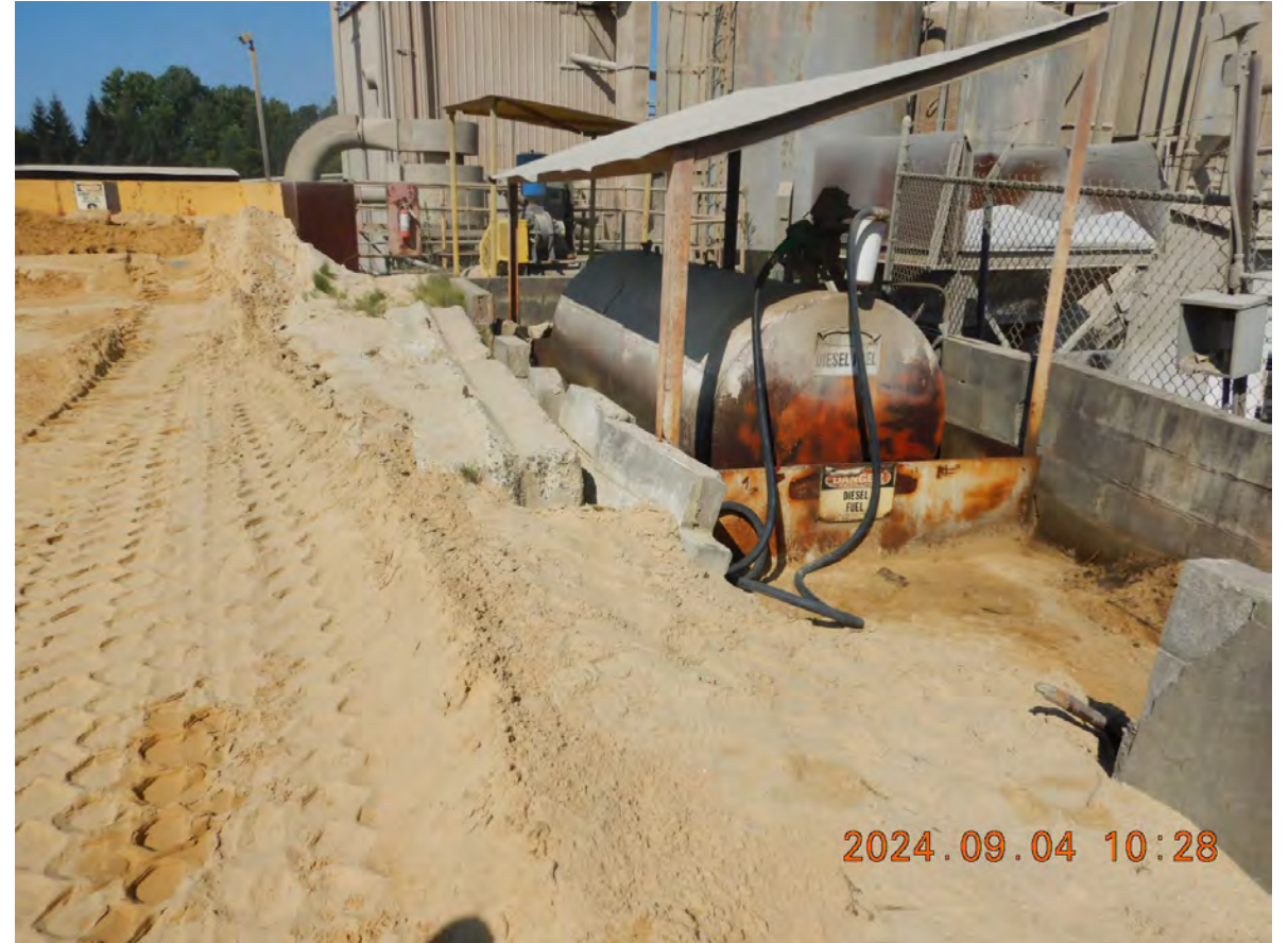
DSCN3752 - Diesel fuel storage used for front end loader; secondary containment in need of repair
