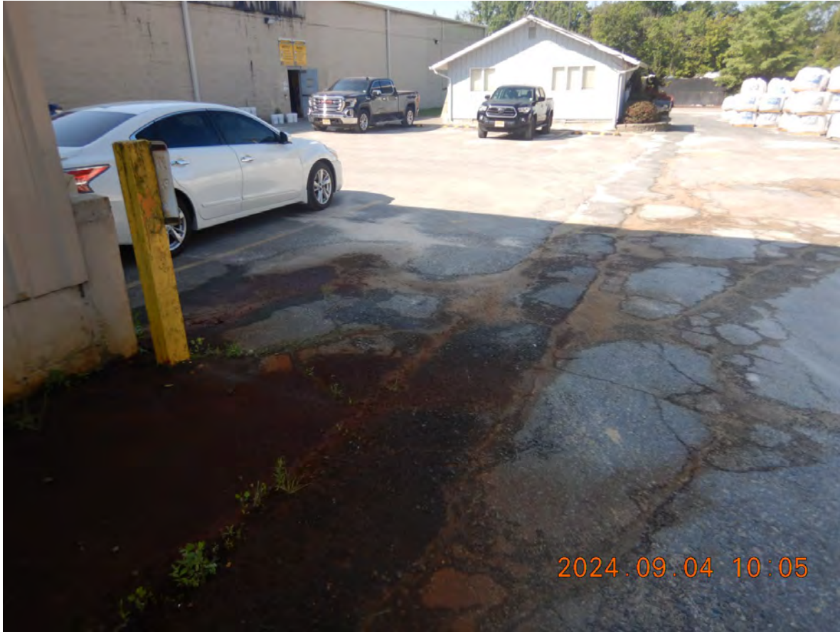
DSCN3682 - Stormwater and source material on pavement in employee parking lot
