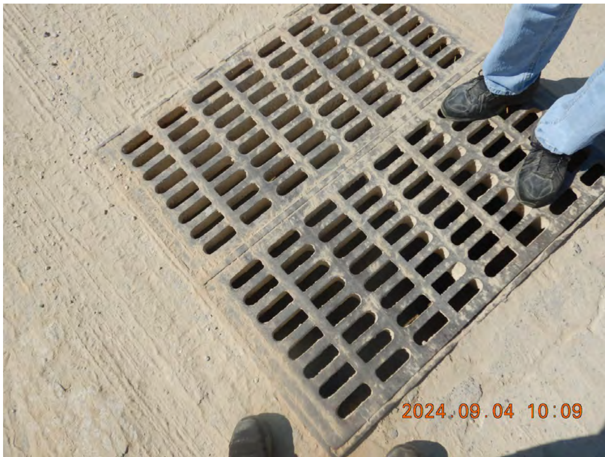
DSCN3703 – Catch basin in the central east portion of the Site
