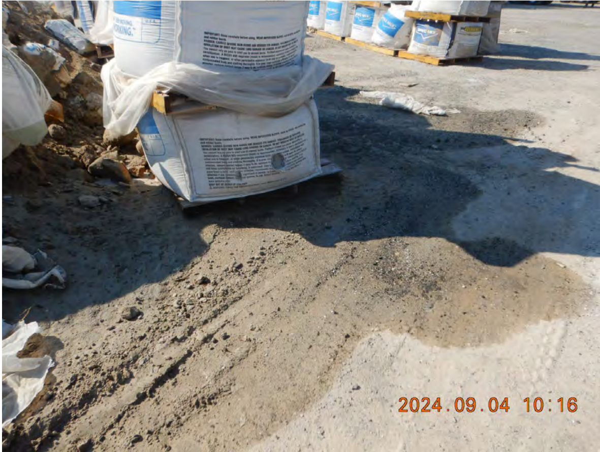
DSCN3731 - Stormwater collecting around material to be recycled
