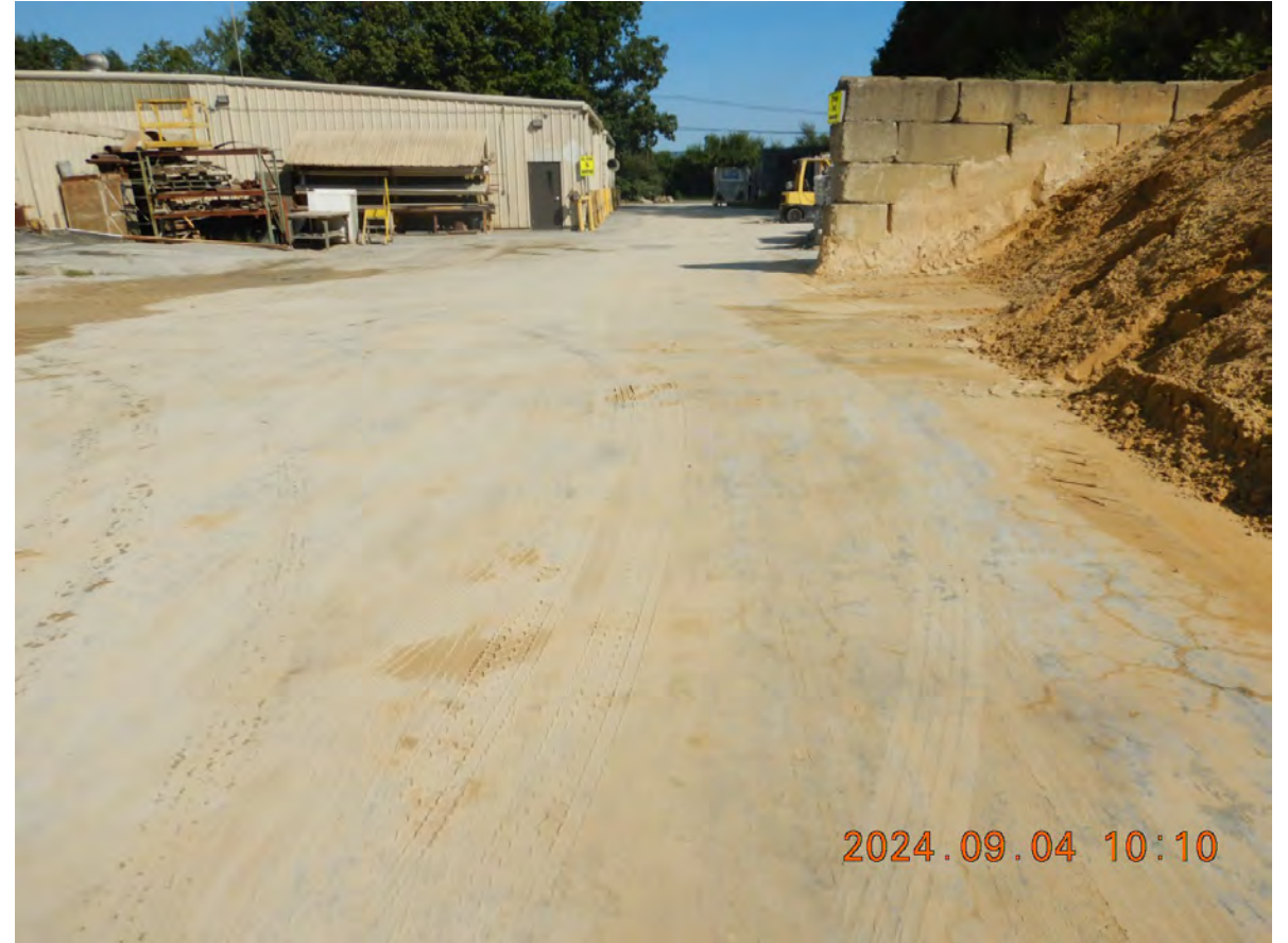
DSCN3712 – Stormwater and source material along drive facing north
