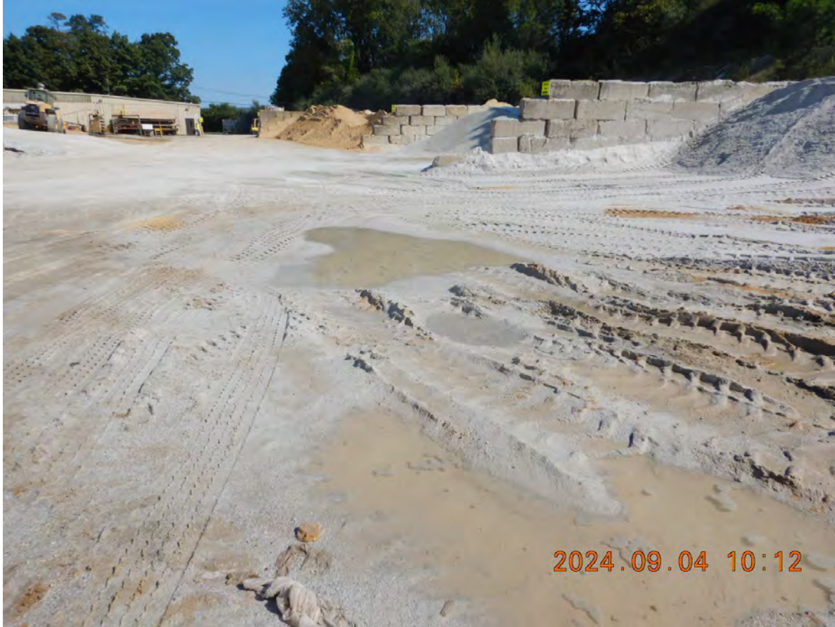
DSCN3719 – Stormwater collecting and pooling on source material; facing north; upgrade of catch basins
