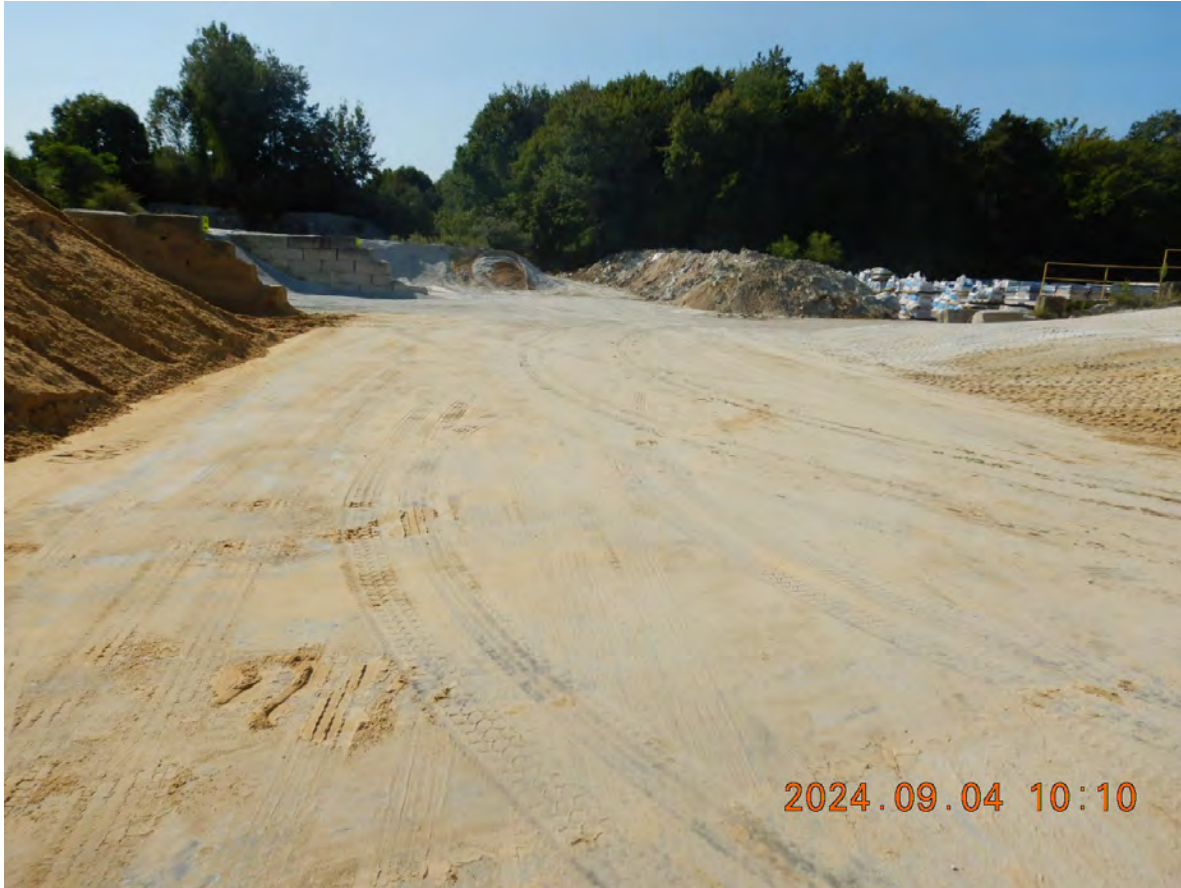
DSCN3711 – East driveway facing south; aggregate bunks, and materials to be recycled
