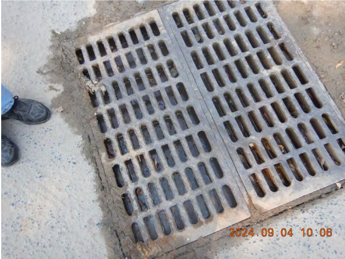
DSCN3688 - Catch basin located at the end of driveway and Gold Mine Rd
