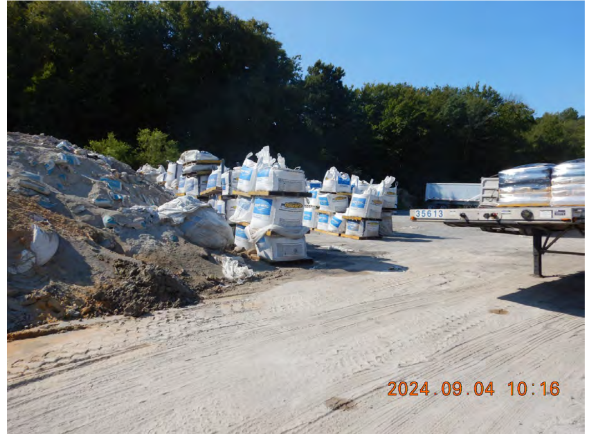
DSCN3730 – Stormwater collecting around material to be recycled
