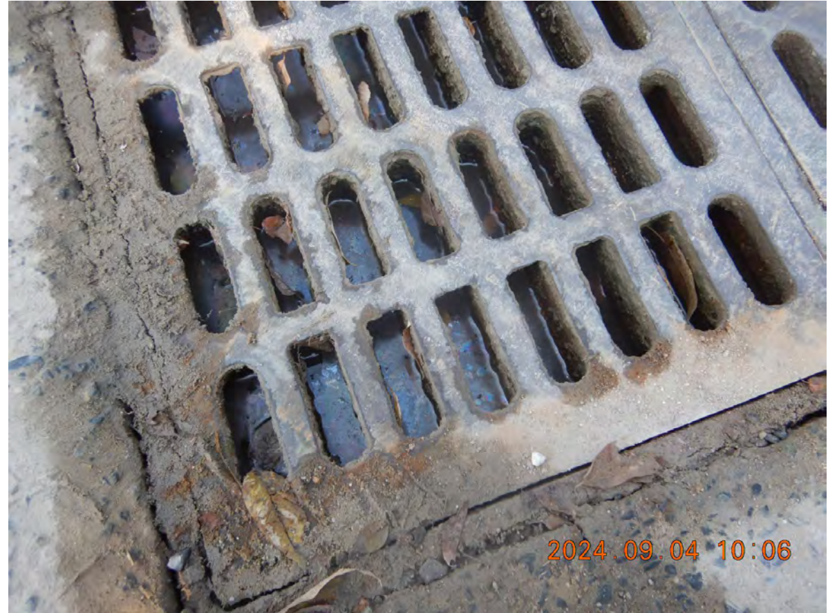
DSCN3689 – Source material, debris, and sheen inside basin
