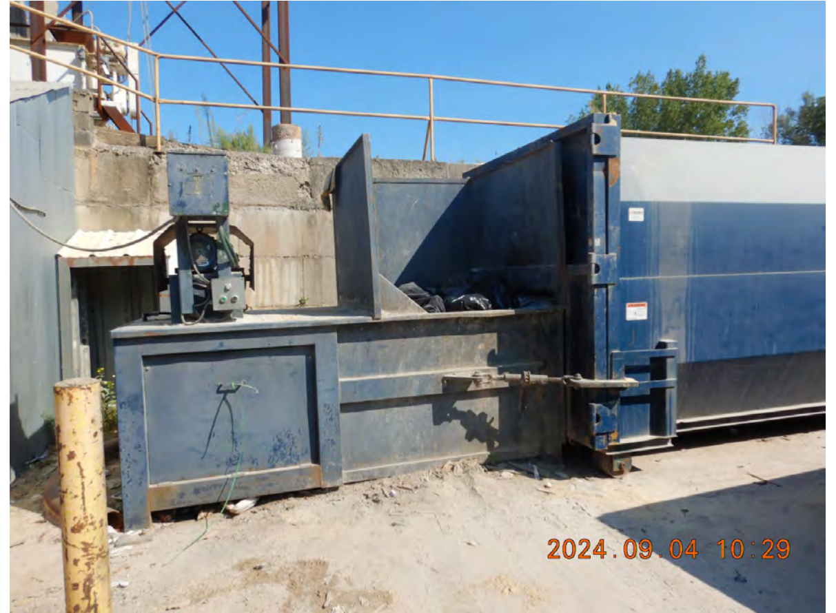
DSCN3761 – Trash compactor in central area of Site
