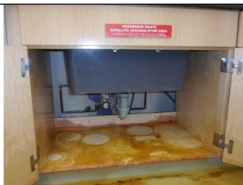
Figure 28: 11:12 AM CP 348 Satellite accumulation area with remnants of cleaned up spill observed.
