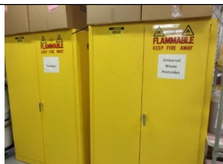
Figure 12: 10:29 AM Oxidizer Storage Two flammable cabinets observed.
