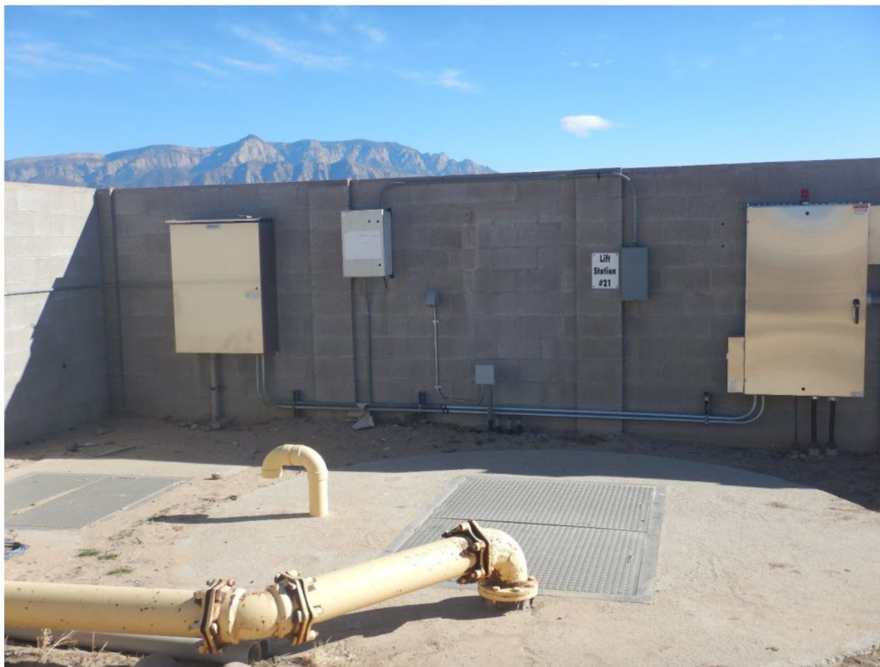
View of Lift Station #21 piping, electrical panels and wet well enclosures inside the former WWTP #3 perimeter fence. (DSCN2746) (12/23/2024) 2:44 PM. Photographed by D. Esparza
