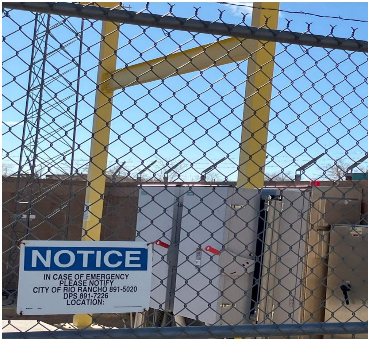
View of minimal warning or electrical hazard signage inside of LS-#15. NOTE: the appearance of a flashing light (alarm) in the center right of photograph located below enclosure. (IMG_0545) Photographed by N. Fuad
