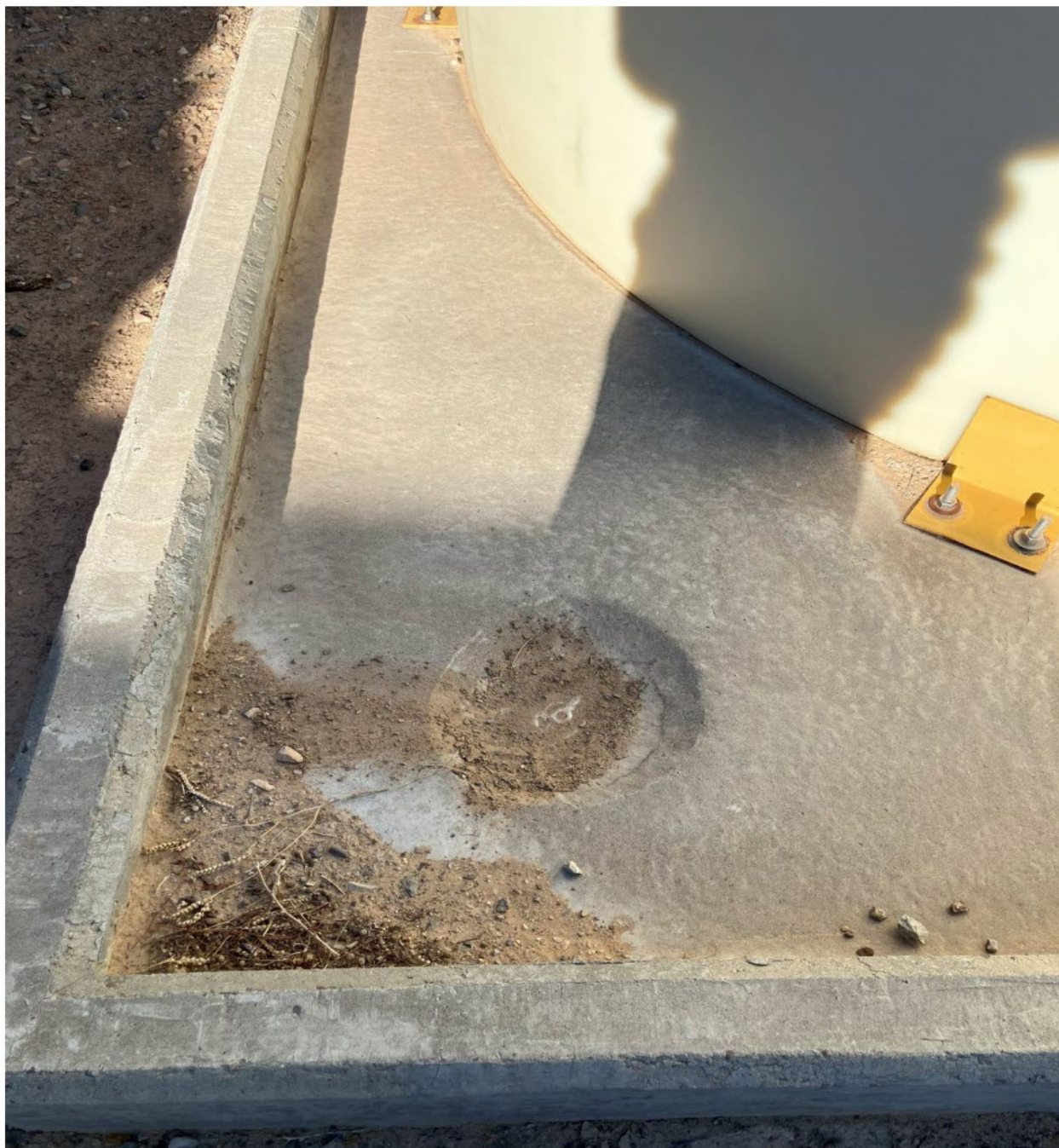
View of the secondary containment obstructed drop drain for the Bioxide tank at LS-#24. (IMG_0576) Photographed by N. Fuad
