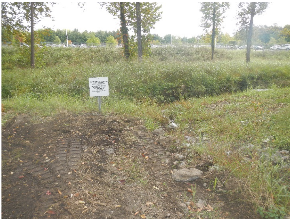
Photo 7. Outfall 002 at Sims Creek.
