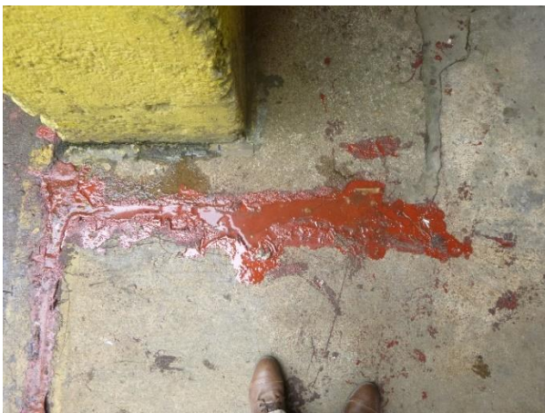
Photograph 56: Worn coating in Area 4 Secondary Containment.
