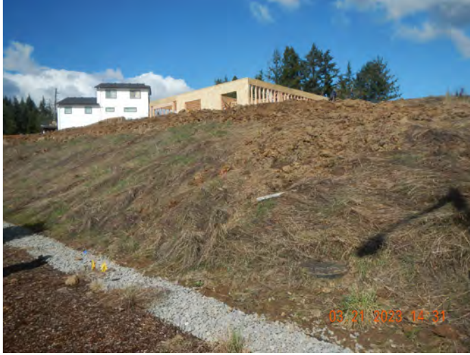
Photo #:17 (DSCN3196) Description: Facing northeast, photo from below lot #40 and lot #41. Exposed soil observed along the southern slope and without perimeter BMPs.
