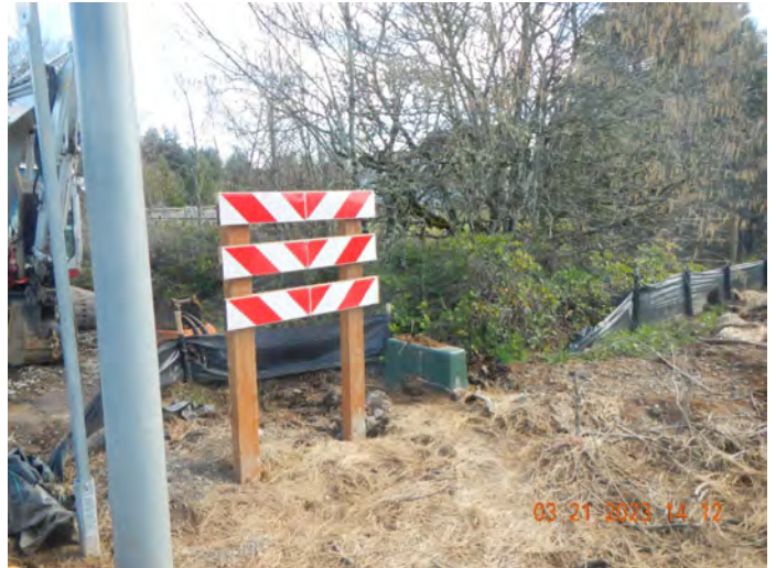
Photo #:12 (DSCN3191) Description: Facing east, photo of the northeast corner of Phase 2. Silt fencing in need of repair.
