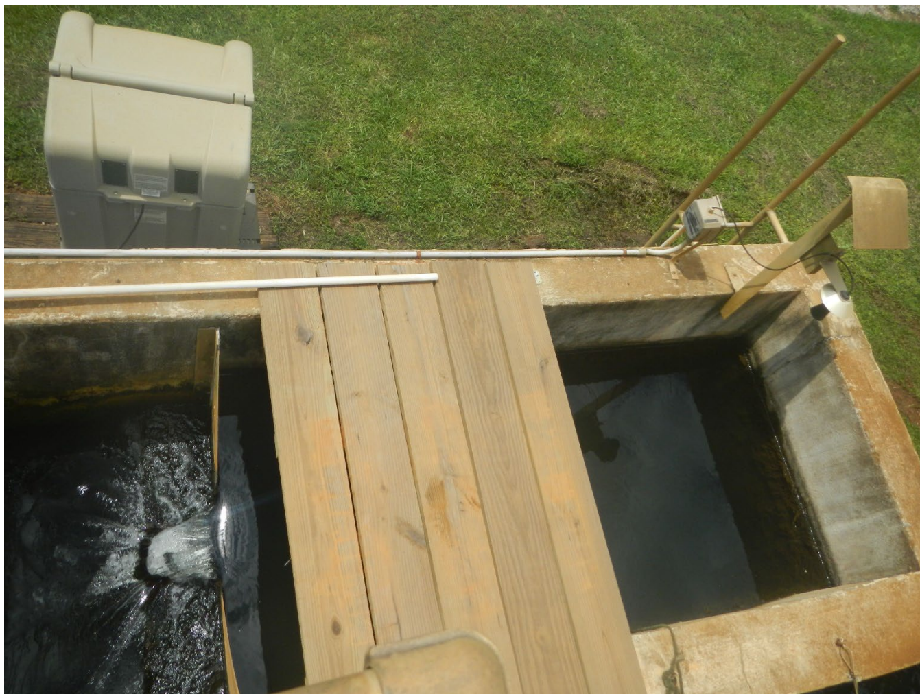
Photo 2: flow measurement (90 degrees V notch Weir) following clarification and disinfection.
