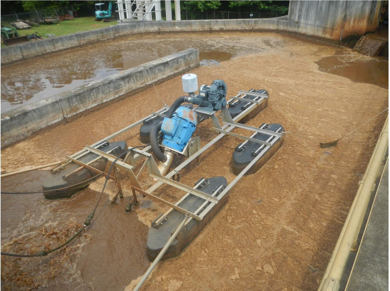
Photo 1: Thick foam observed in aeration basin.
