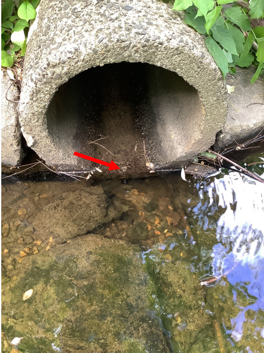
EastST (photo taken 5/24 at 10:51 AM): Outfall located at the southern end of the Kingdom of Jehovah's Witnesses parking lot, flowing into the stream coming from Searles Pond. Sample point is indicated by a red arrow.
