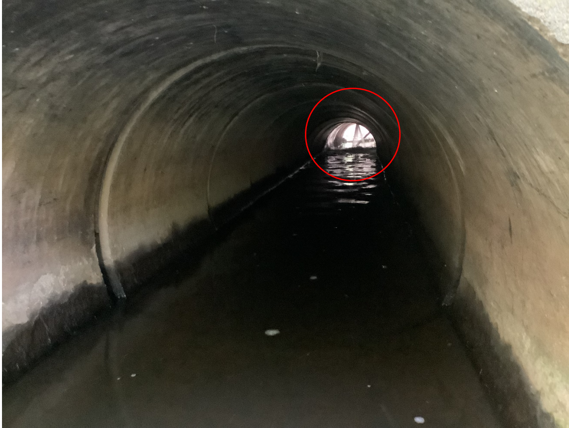
Renfrew2 (photo taken 5/24 at 08:48 AM): Downstream view of unidentified discharge spraying into Bare Meadow Brook from the top of the culvert, indicated by a red circle.
