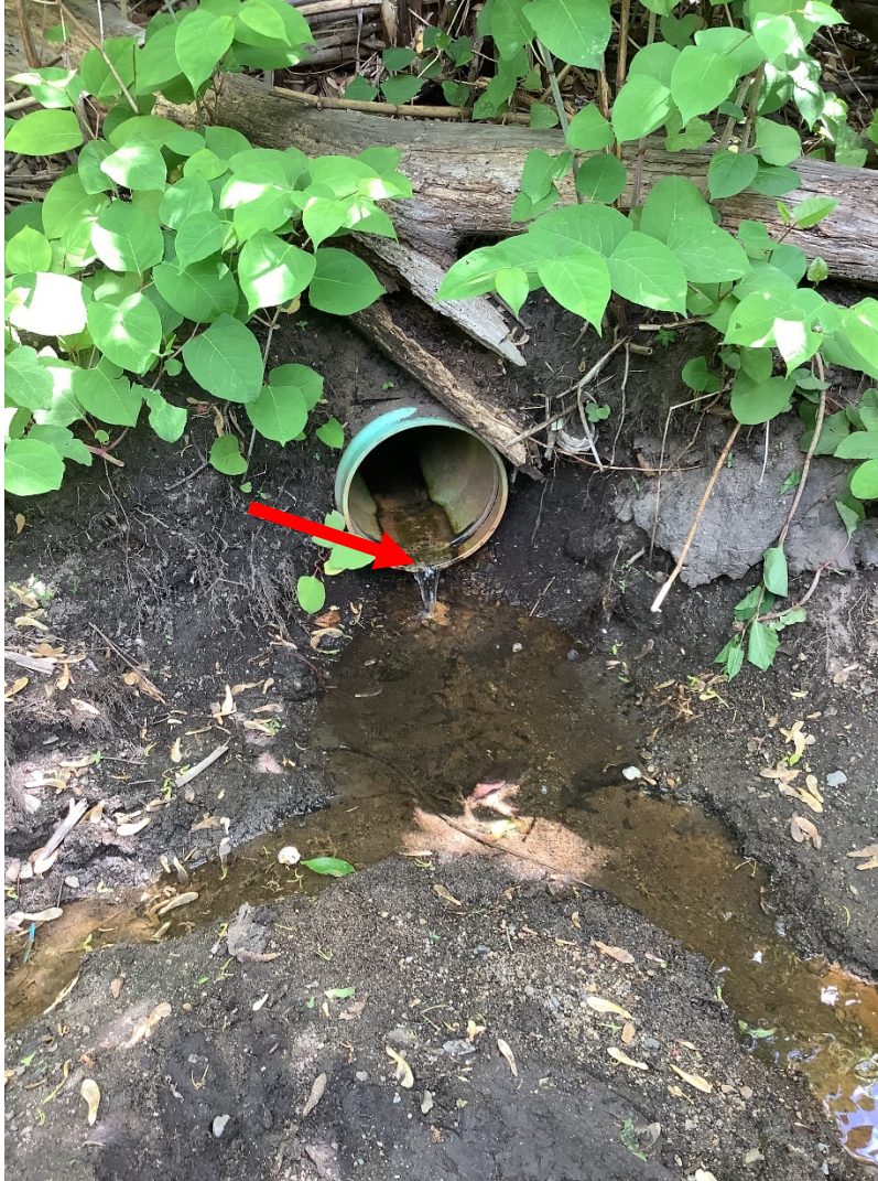
Horne (photo taken 5/24 at 12:27 PM): Outfall located at the northwest corner of Horne Street, just north of the intersection with Huse Road, flowing into the Spickett River. Note the orange staining of the pipe and sediment. Sample point is indicated by a red arrow.
