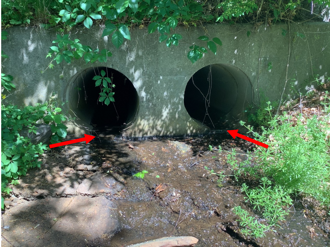
Outfall 1A & 1B (from left to right) (photo taken 5/25 at 10:09 AM): Pair of outfalls located within the Pride's Crossing complex flowing into the Merrimack River. Sample points are indicated by red arrows.
