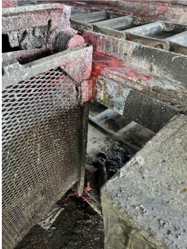
View of liquids and solids collecting beneath the conveyor line that leads into the furnace. {Photograph 15, Attachment 1}
