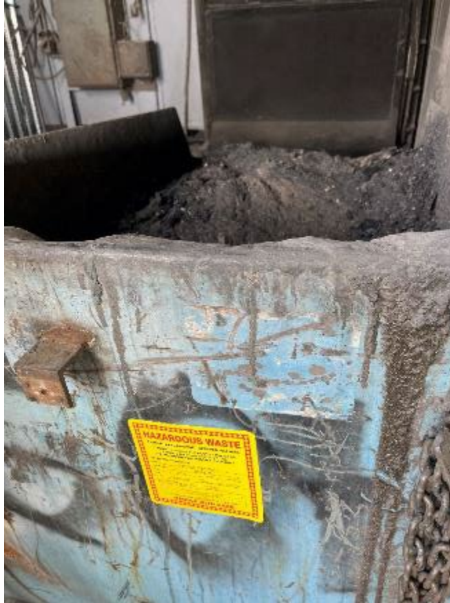
View of furnace ash hopper located near the furnace. The hazardous waste label lists waste codes D001, F003, and F005, which are not accurate for the potential hazards for this waste stream. {Photograph 11, Attachment 1}
