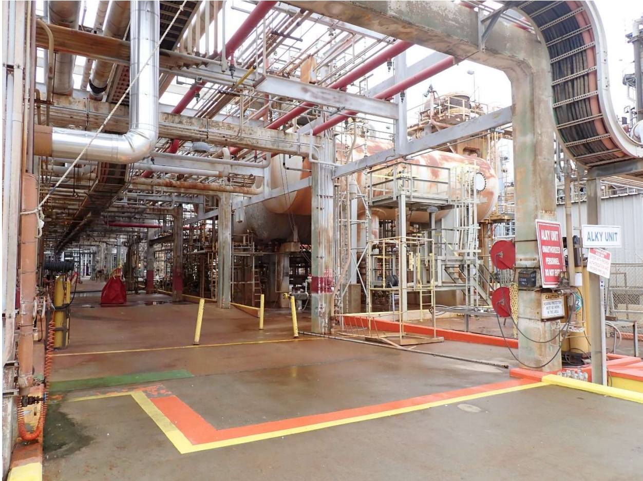
Photograph 3 - File: PB130003.JPG HF Truck Unloading Station.
