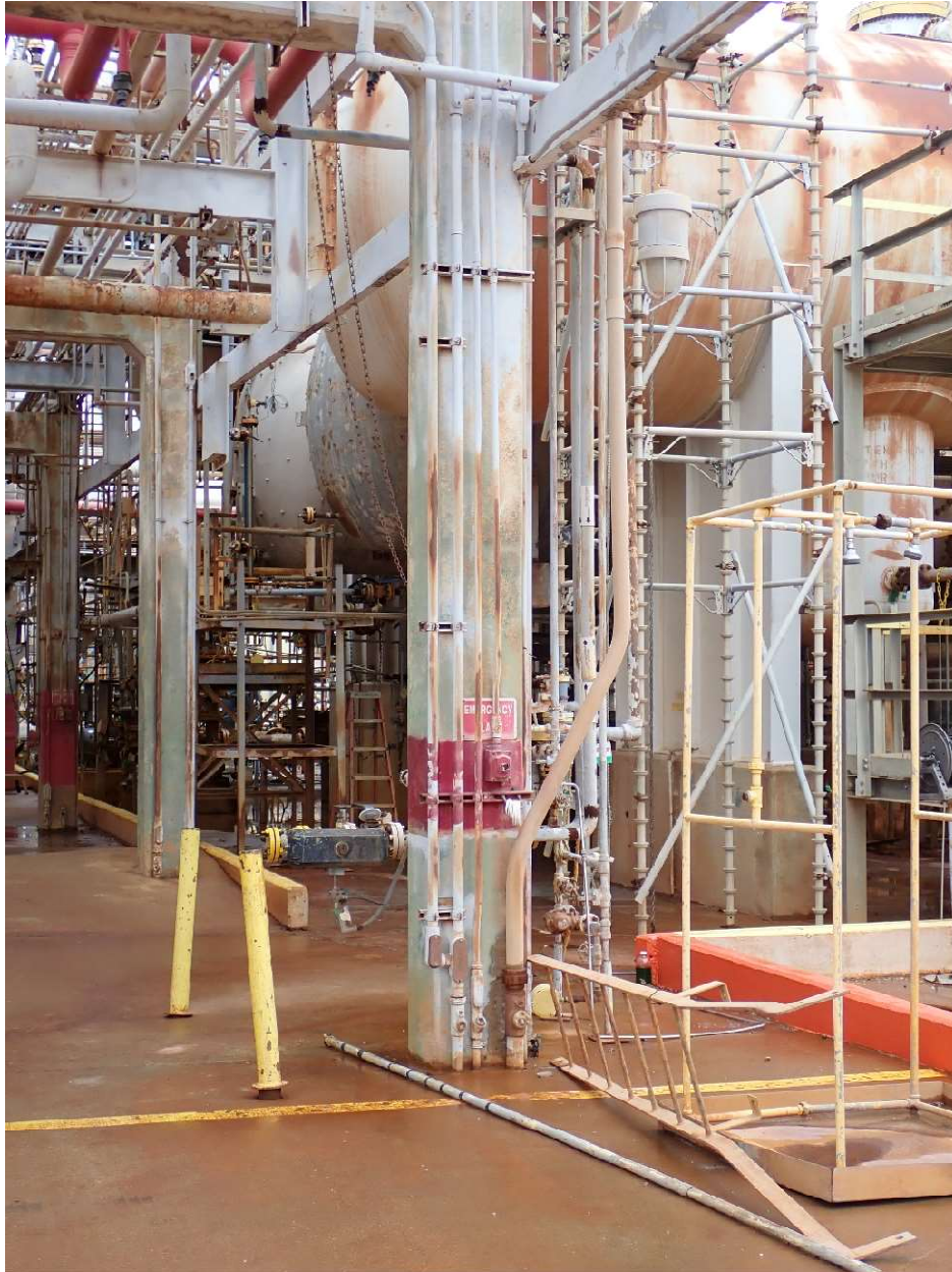
Photograph 5 - File: PB130005.JPG HF Truck Unloading Connection Point.
