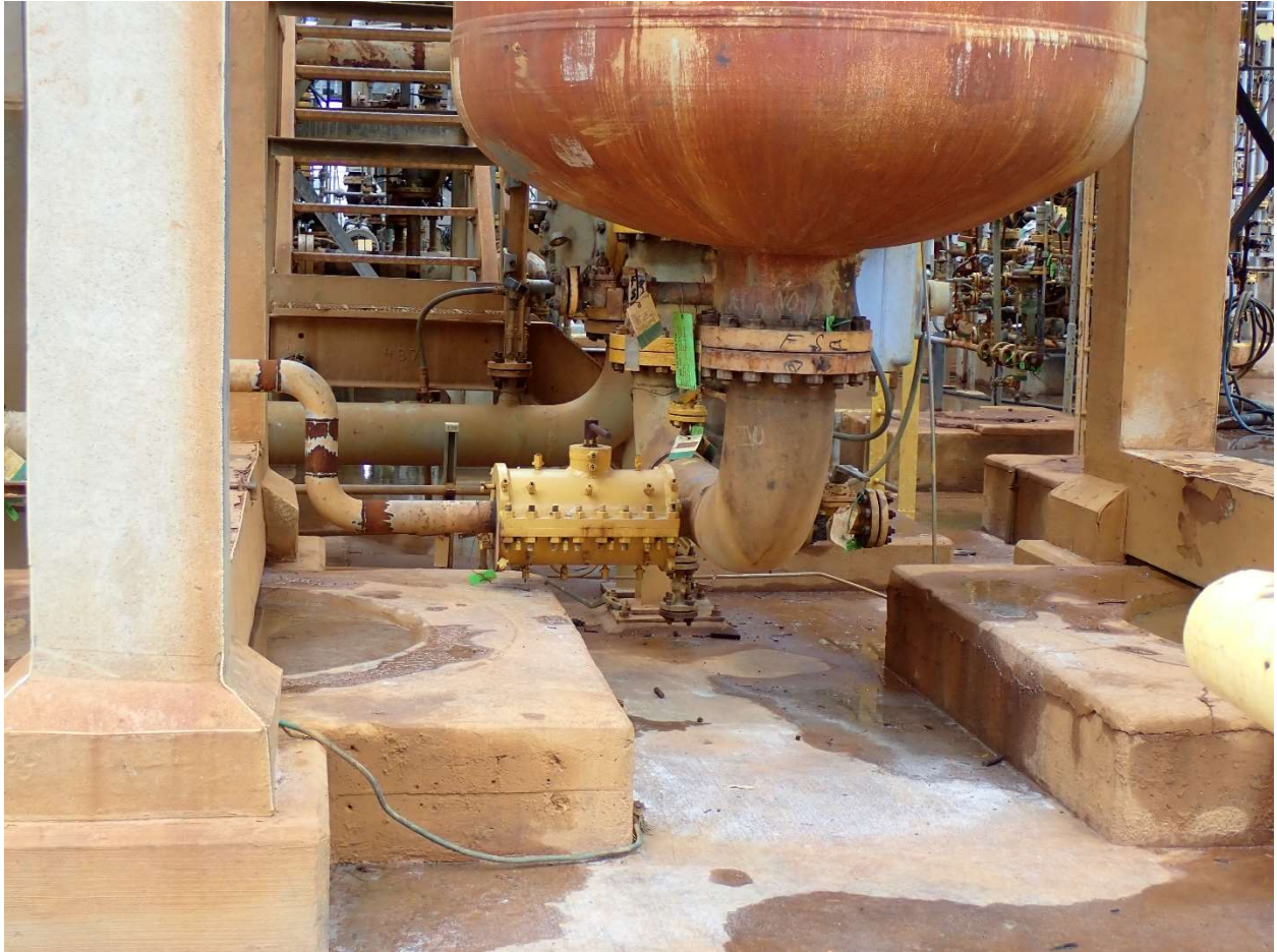
Photograph 6 - File: PB130006.JPG Temporary Clamp under Tank E-621.
