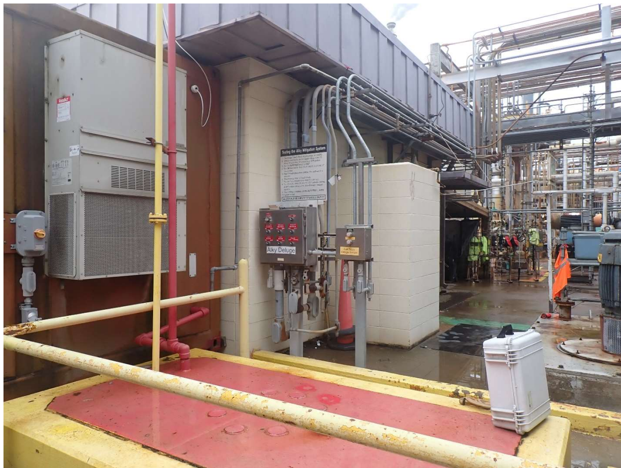
Photograph 1 - File: PB130001.JPG Alky Mitigation Control System near the Alkylation Unit Change House.
