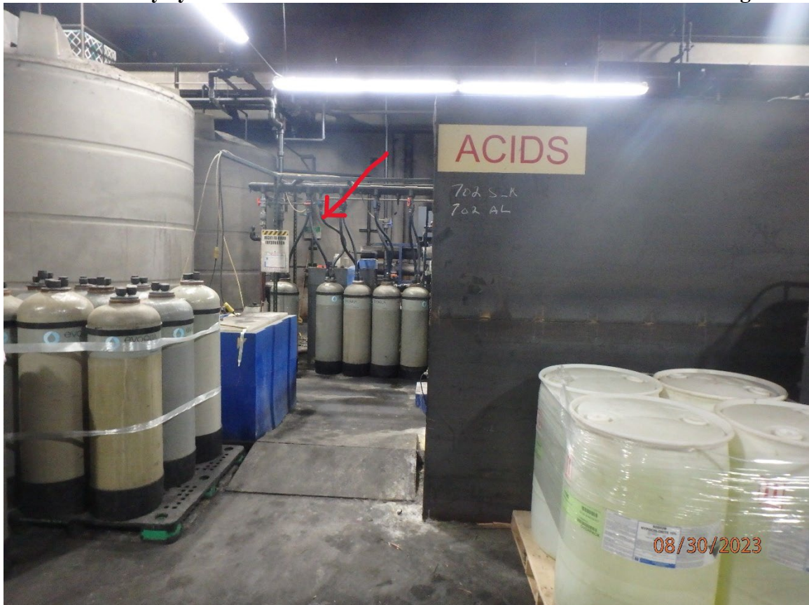
Photo 4. Safety eyewash/shower location nearest to the Acids & Bases Storage
