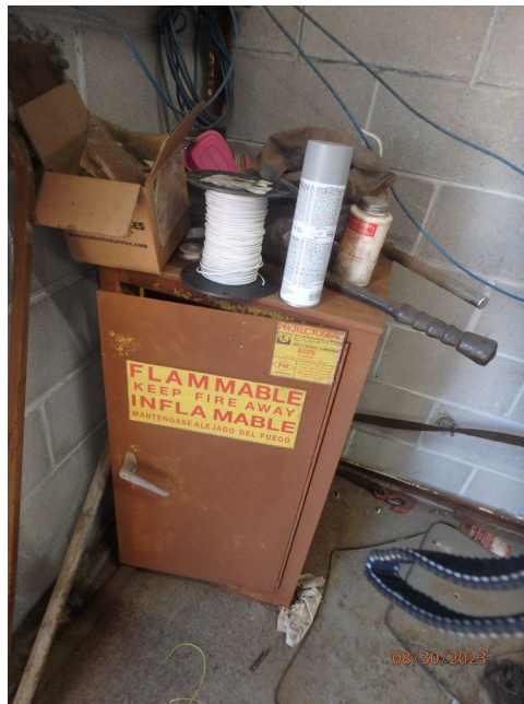
Photo 3. Inside Chlorine Building
