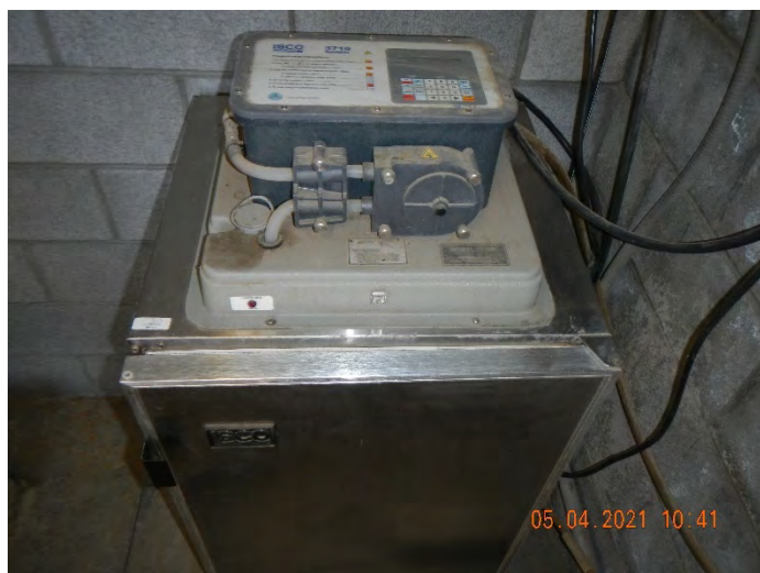
Photo #:03 (DSCN2109) Description: Near the headworks, photo of ISCO 3710 refrigerated influent sampler.
