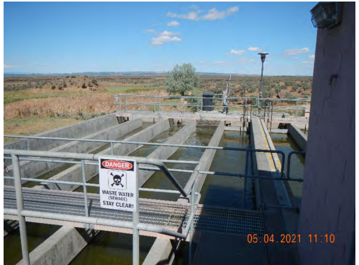
Photo #:08 (DSCN2116) Description: Facing north, photo of the chlorine contact chamber.
