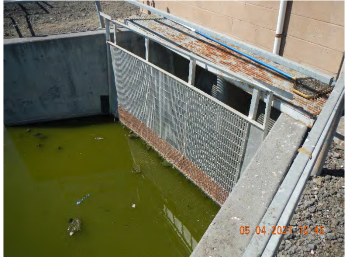
Photo #:06 (DSCN2112) Description: Facing south, photo of manual coarse screen located at the end of the open channel.
