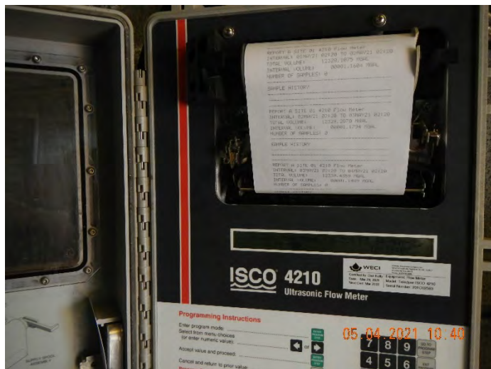
Photo #:01 (DSCN2108) Description: Photo of the ISCO 4210 Flow Meter control panel and recording log. Flow was reading 1.1MGD at the time of the photo.
