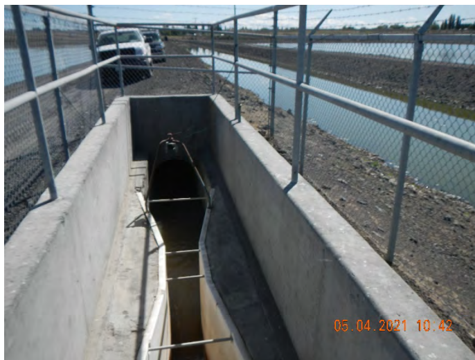
Photo #:02 (DSCN2110) Description: Facing east, photo of the influent weir and flow meter.
