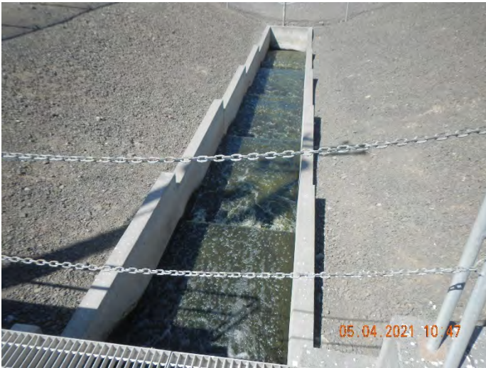
Photo #:07 (DSCN2114) Description: Facing west, photo of the cascade aeration channel (concrete step aerator).
