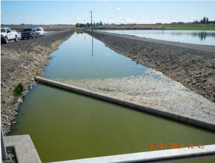
Photo #:05 (DSCN2111) Description: Facing east, photo of the open channel that receives wastewater from the two primary lagoons.
