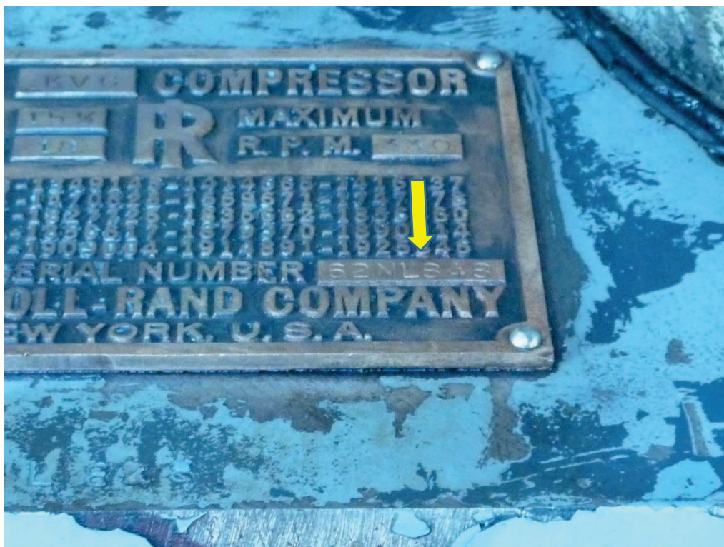
Faceplate of Ingersoll-Rand 62K VG, 660 bhp Reciprocating Compressor Engine – Unit 3 with Serial Number: 62NL848 (emphasis added)
