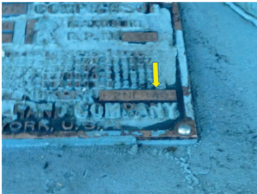
Faceplate of Ingersoll-Rand 62K VG, 660 bhp Reciprocating Compressor Engine – Unit 4 with Serial Number: 62NL849 (emphasis added)
