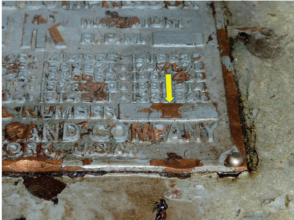
Faceplate of Ingersoll-Rand 62K VG, 660 bhp Reciprocating Compressor Engine – Unit 1 with Serial Number: 62NL846 (emphasis added)
