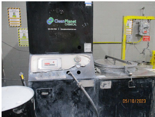
Photo 13: Clean Planet Chemical Xylene Recycler.
