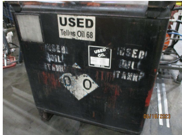
Photo 8: 250-gallon double-walled AST labeled “Used Oil”.
