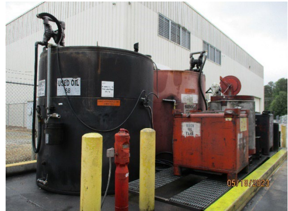
Photo 22: Used Oil Storage Area 1
