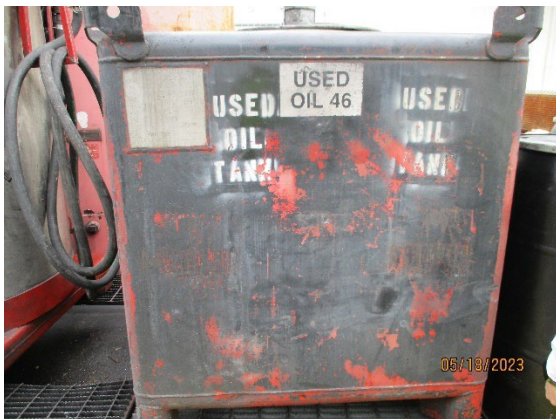
Photo 23: 350-gallon AST labeled "Used Oil" in Used Oil Storage Area 1.
