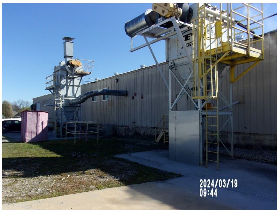
Photograph 2: Picture of Facility Baghouses.
