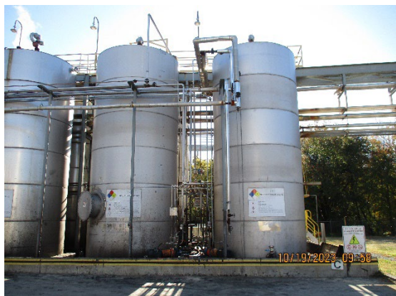
Photo 9: Process Tanks C-9 (Dirty Mixed Solvents) and C11 (Recovered Mixed Solvents).
