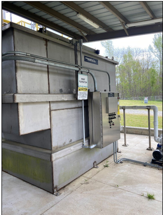
Photo 6: Cloth media filter (not in service).
