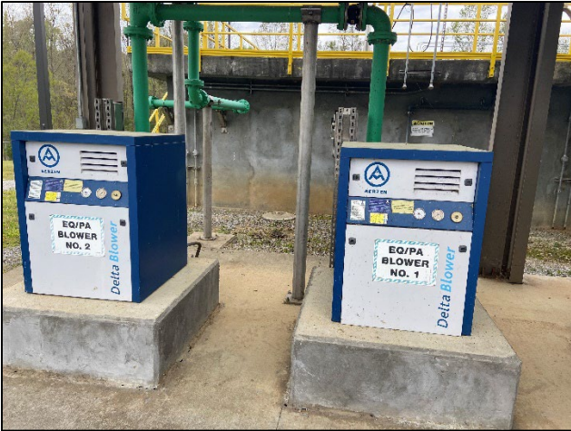
Photo 1. Equalization basin blowers.
