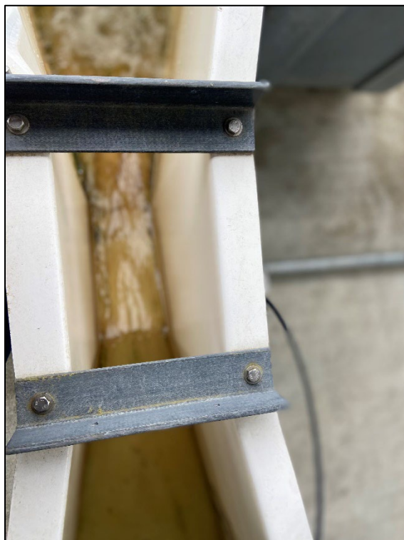
Photo 8: Effluent Parshall flume.
