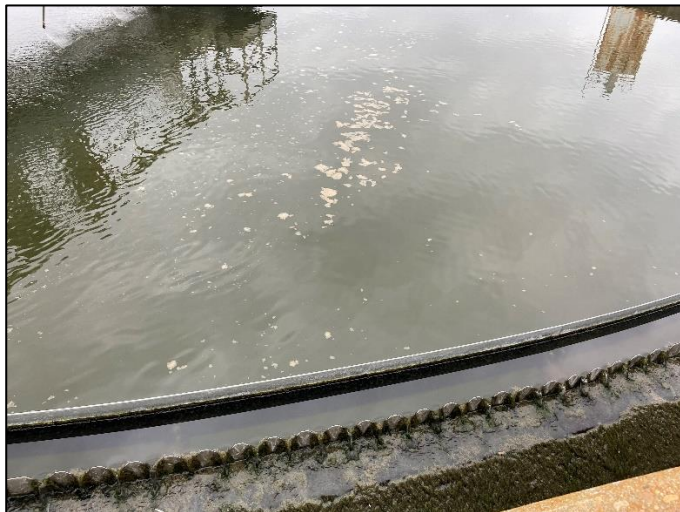
Photo 3: Clarifier #2 (note algae on weirs).
