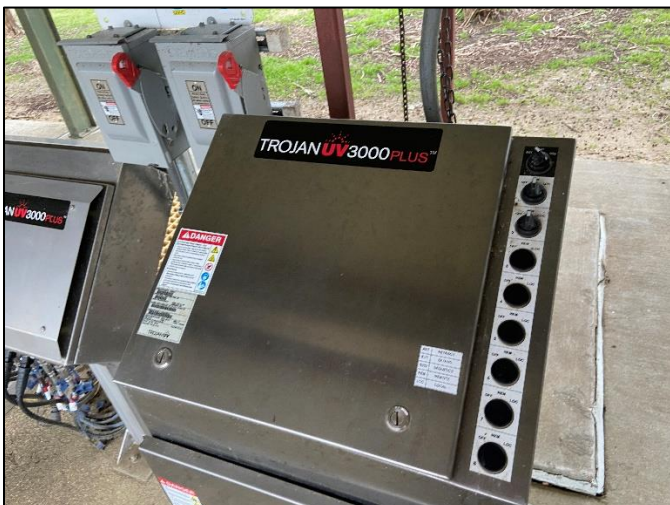
Photo 5: UV disinfection system.
