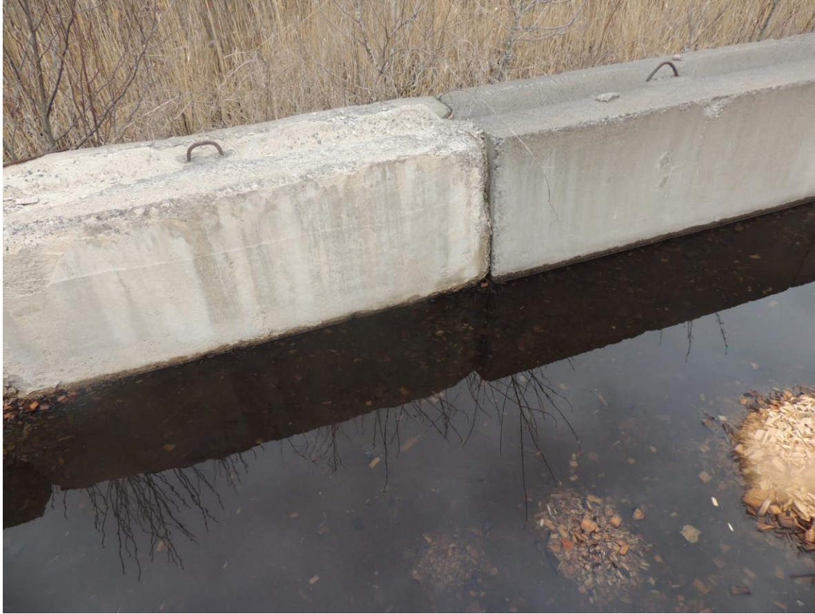
DSCN4030 – Block walls southwest portion of the Site – wet area with phragmites downgradient from the wall
