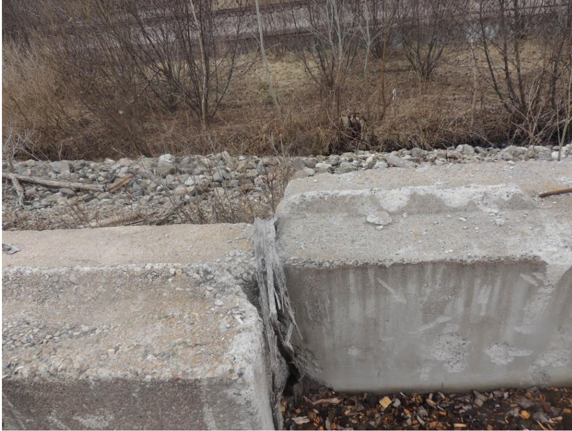
DSCN4026 – Gaps in the block wall around the facility southwest corner of Site
