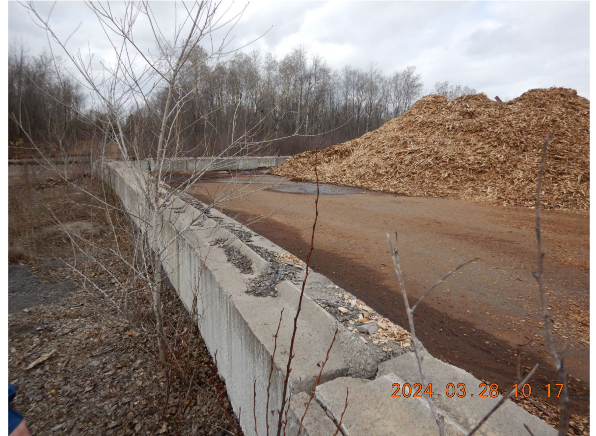
DSCN2707 - Stormwater runoff on S lot of Site. There are small gaps in the block wall where stormwater could flow out of.
