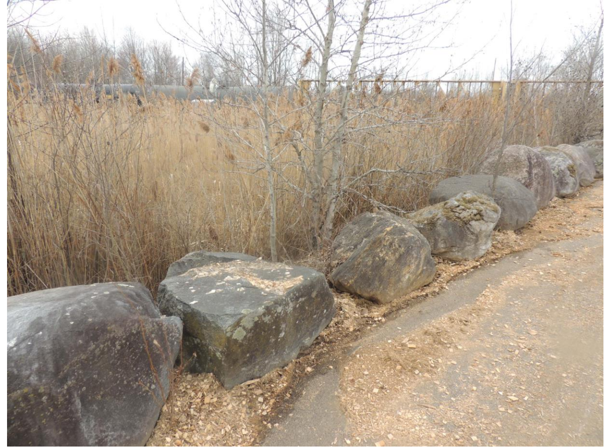
DSCN4037 – Gap in block wall on the southwest portion of the Site – with woodchip accumulation
