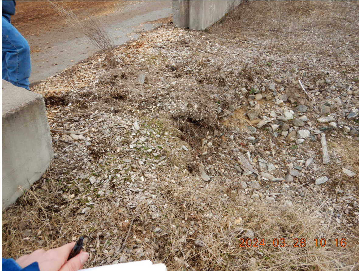
DSCN2703 - Stormwater flow path and erosion on S lot of Site
