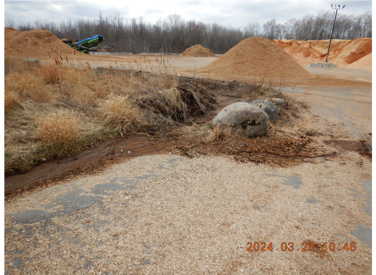
DSCN2750 - Condensate runoff from manufacturing equipment
