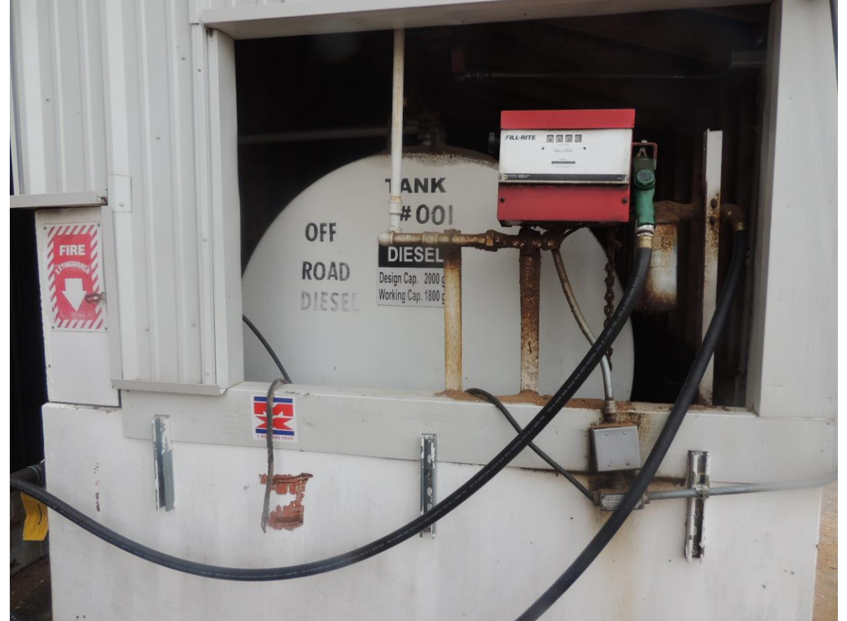
DSCN4039 – 2,000 gallon off road diesel tank covered and in secondary containment
