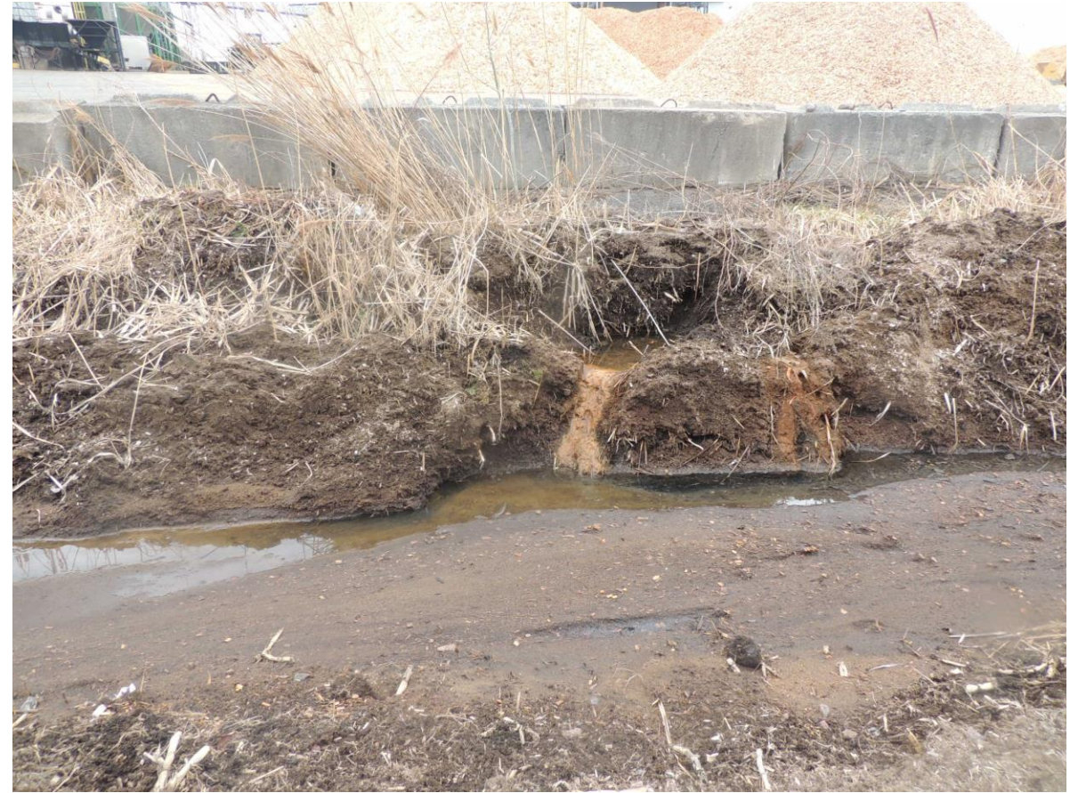
DSCN3995 Stormwater outfall on the West of Site near CSX tracks; Stormwater from catch basin located near the South corner of the packaging warehouse. The outfall is not visible (and needs to be cleaned). Channel for stormwater flow also seen
