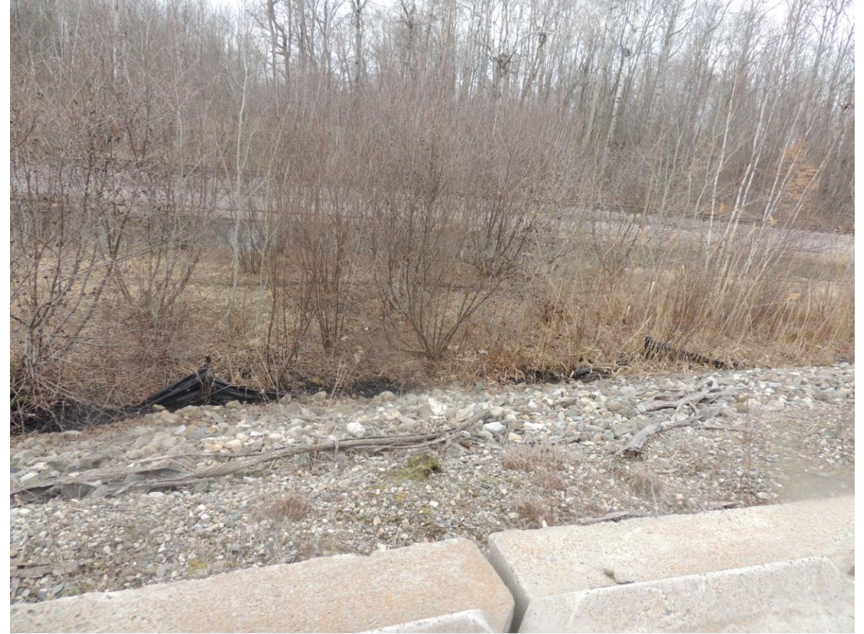
DSCN4027 – Remnants of silt fencing seen on the slope down from Facility (SW side)
