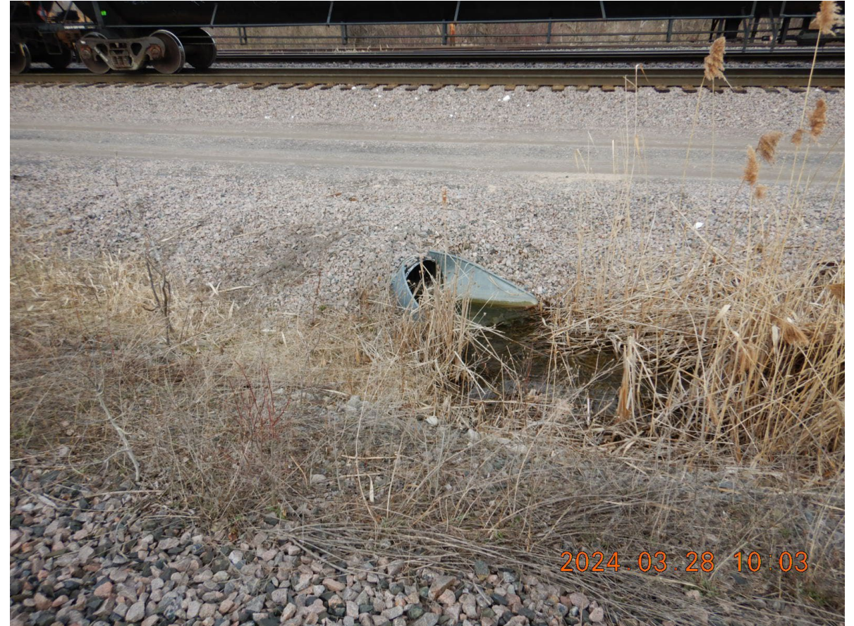
DSCN2686 - Stormwater drainage on the W side of materials and waste storage
