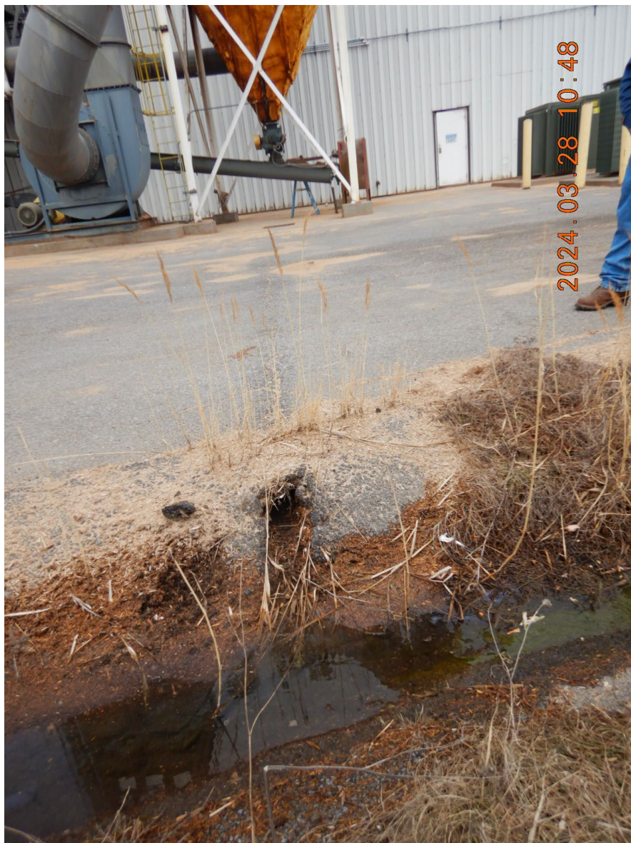
DSCN2757 - Drainage with water that gets flow from Catch Basin #3
