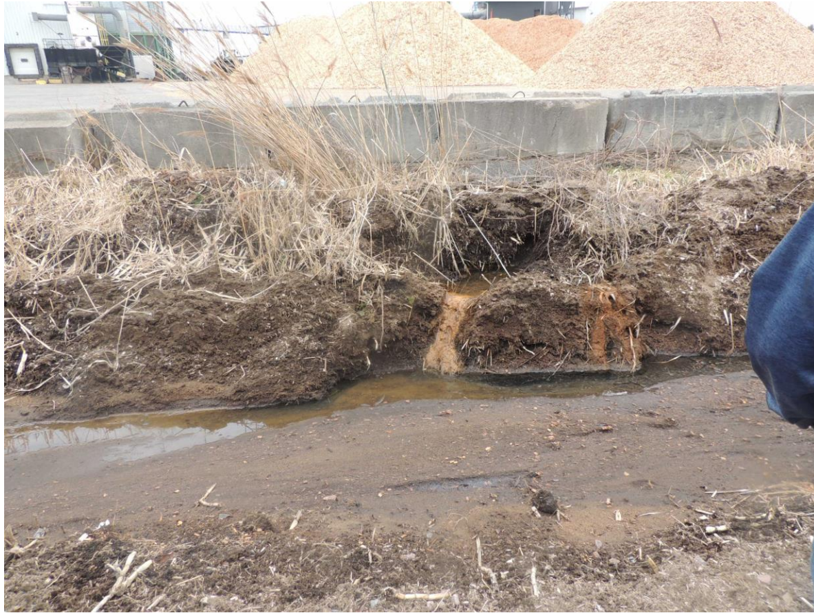
DSCN3994 - Stormwater outfall on the West of Site near CSX tracks; Stormwater from catch basin located near the South corner of the packaging warehouse. The outfall is not visible (and needs to be cleaned). Channel for stormwater flow also seen
