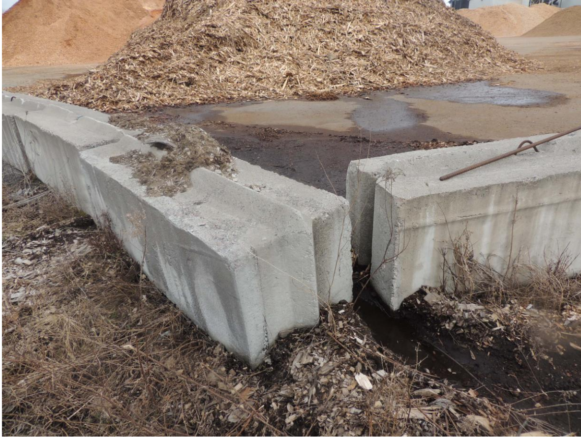
DSCN4020 – Drainage pathway for stormwater to flow from woodchip piles through the block walls on the southeast portion of the Site, area is wet
