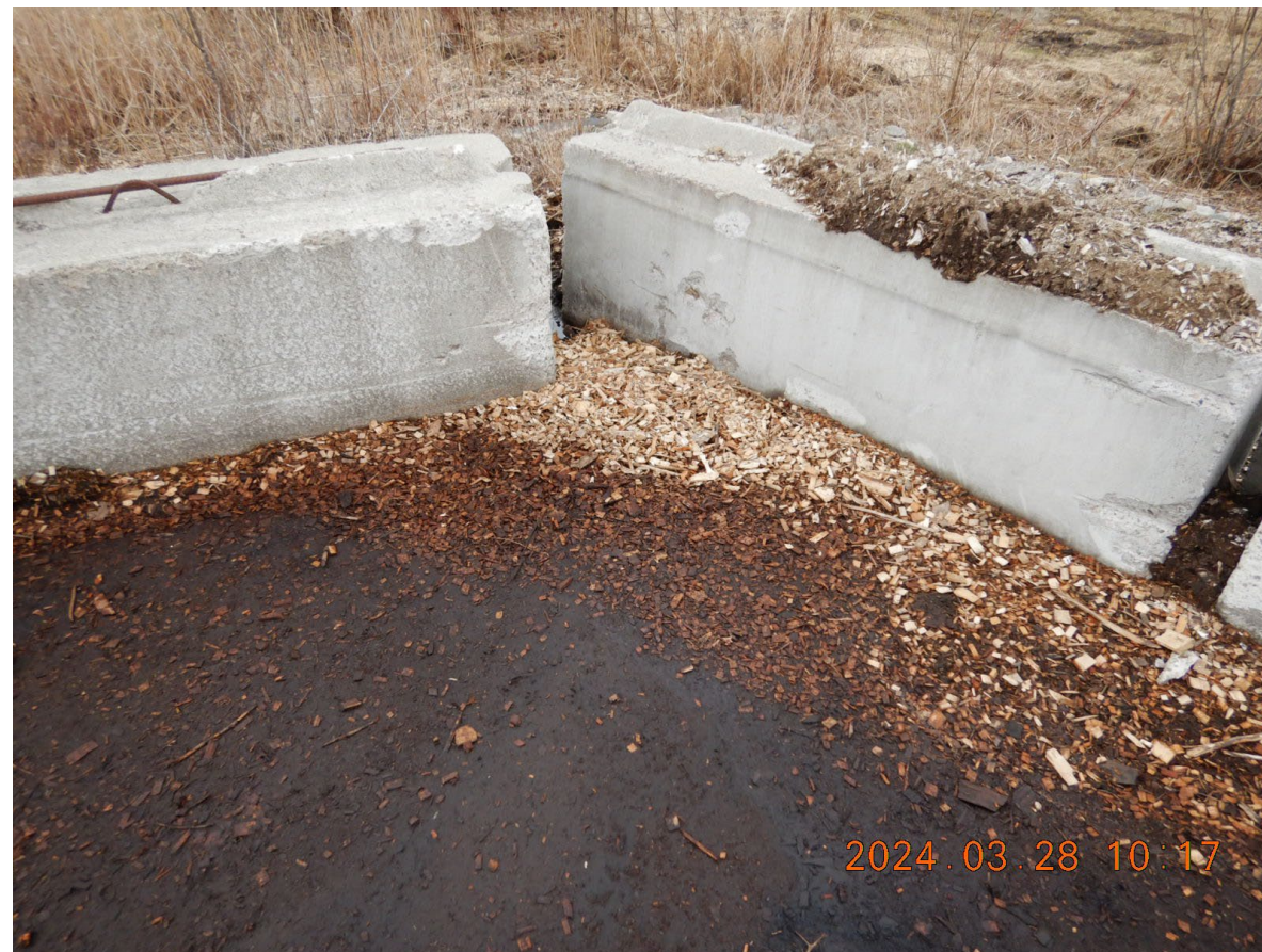
DSCN2709 - Stormwater runoff on S lot of Site
