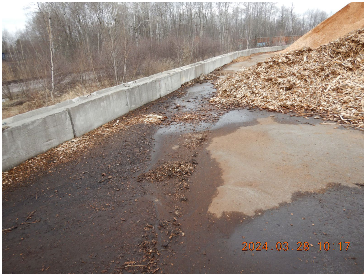
DSCN2708 - Stormwater runoff on S lot of Site
