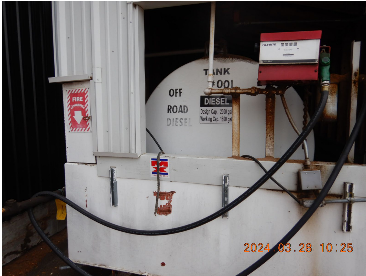
DSCN2722 - Diesel Tank located near woodchip unloading and loading in central area of Site
