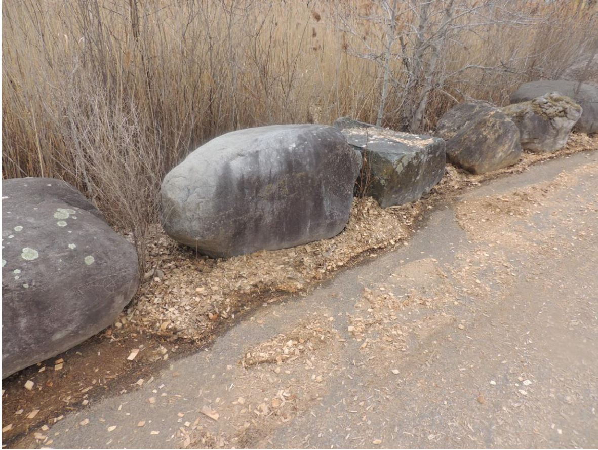
DSCN4036 - Gap in block wall on the southwest portion of the Site – woodchip accumulation
