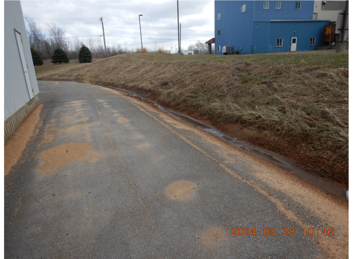
DSCN2752 - Stormwater drainage on S side of pellet manufacturing building
