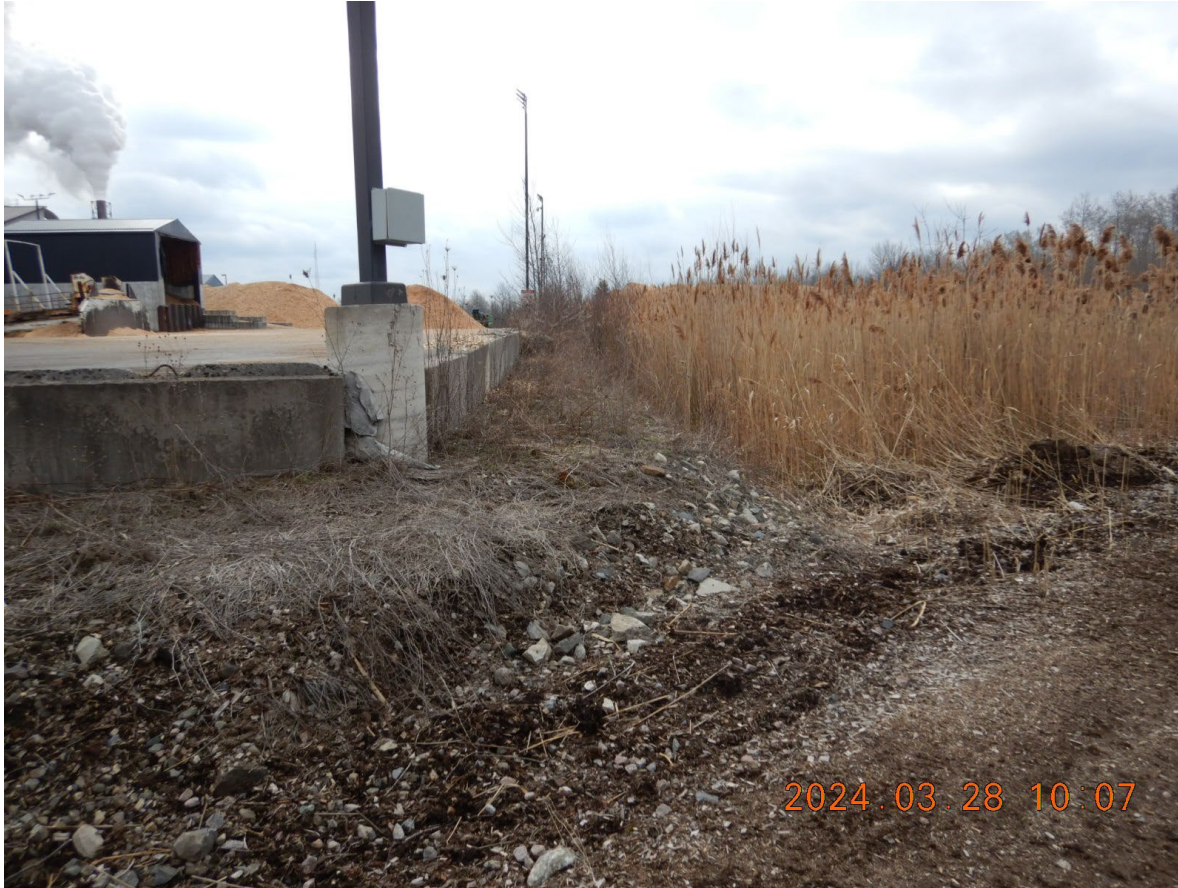
DSCN2690 - Stormwater drainage of furtherest W corner of Site
