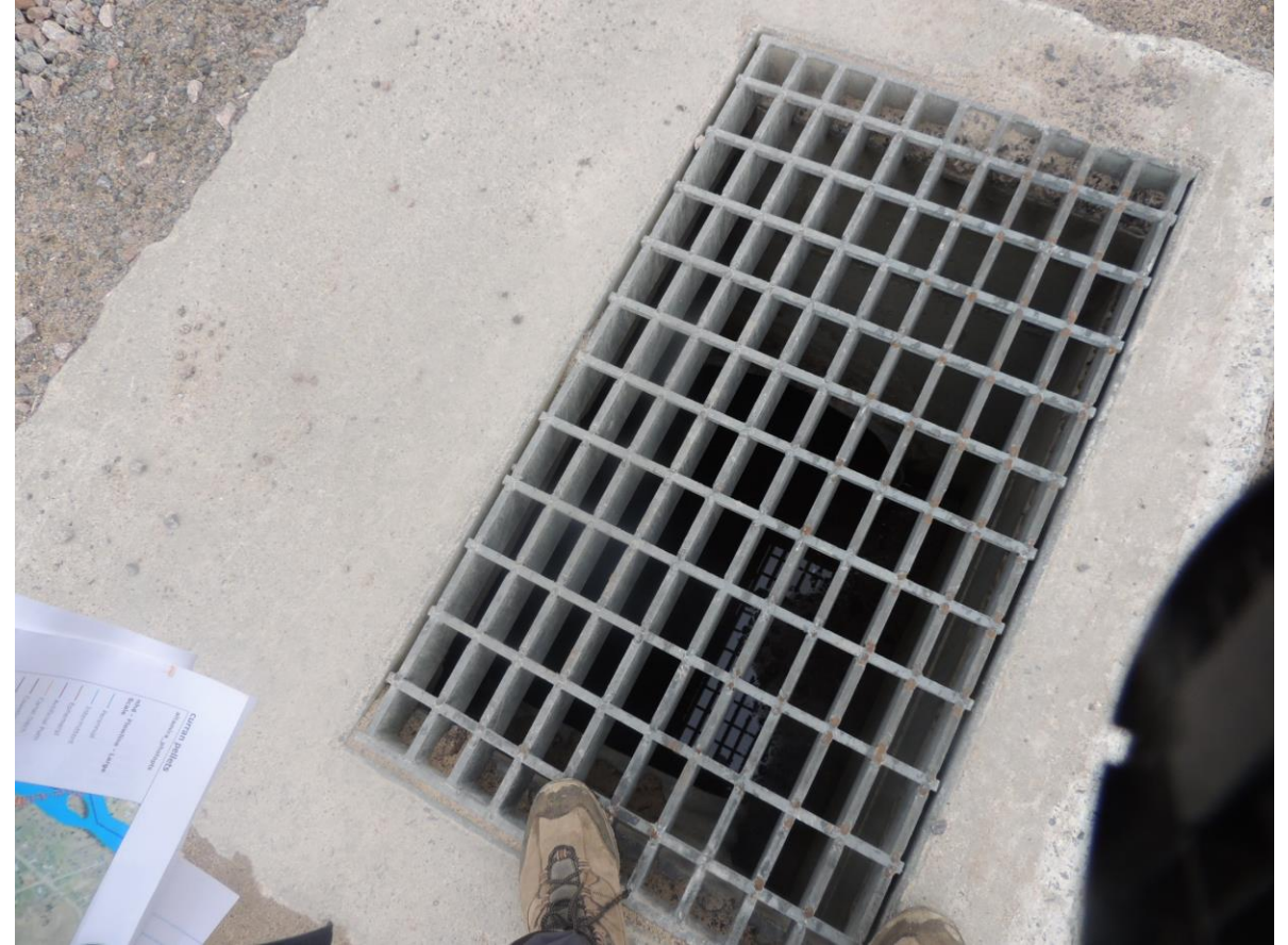
DSCN3999 - Catch basin located on railroad property along Western edge of Site, stormwater piping seen in the storm sewer
