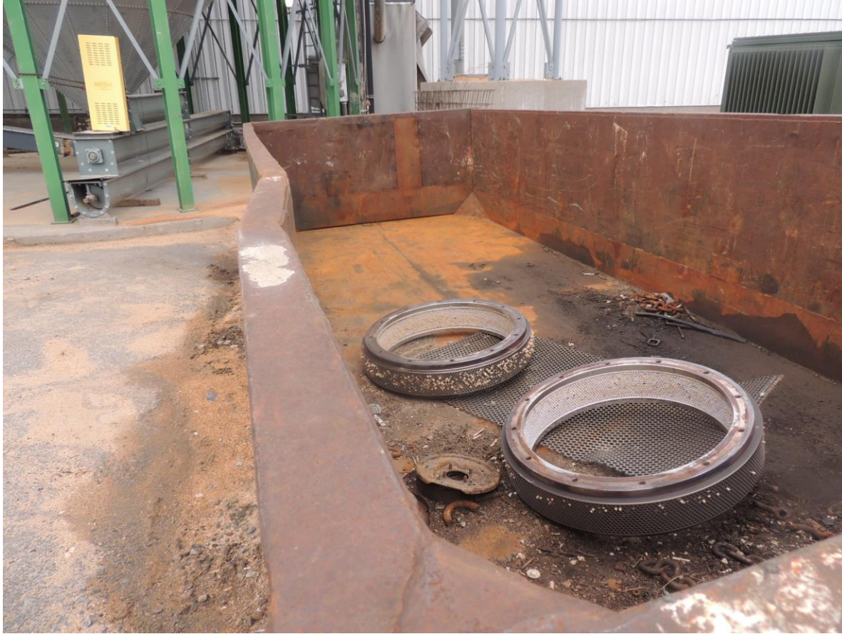
DSCN3990 – Scrap metal dumpster - uncovered
