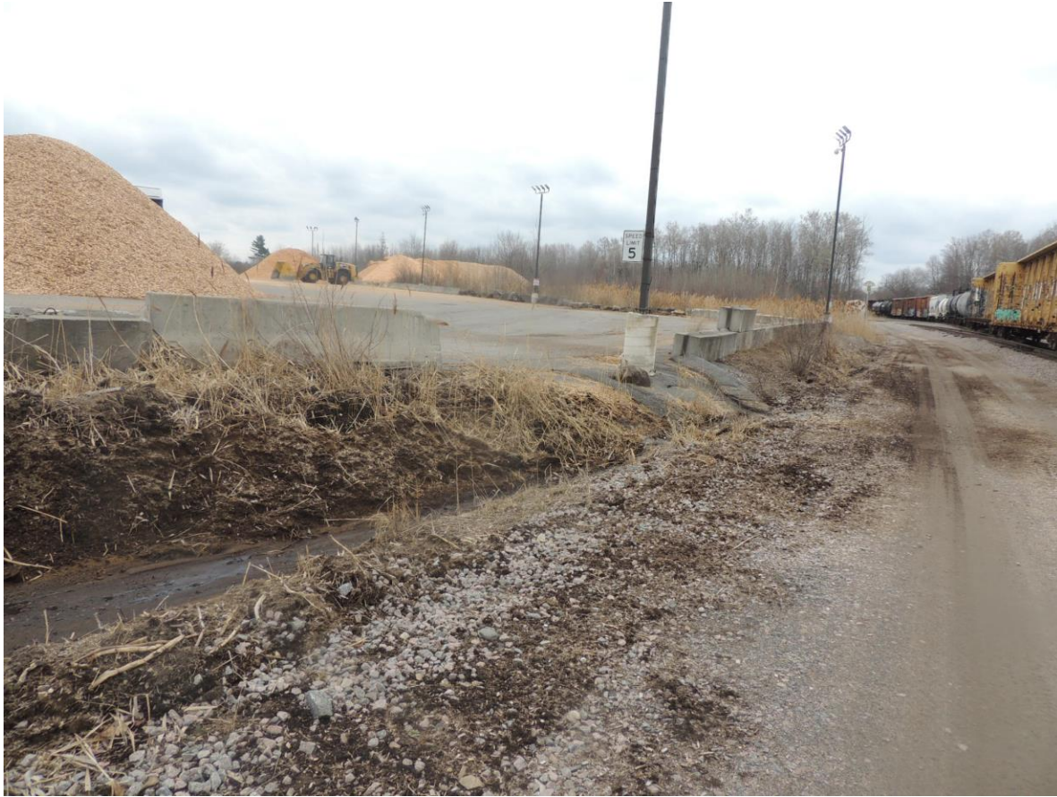
DSCN3996 – Storm channel along western portion of the Site adjacent to the CSX rail line and a break in block wall that would allow stormwater flow off the site.
