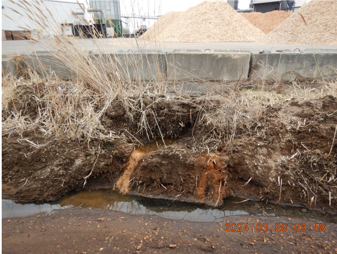
DSCN2671 - Stormwater outfall on the W edge of Site; Stormwater from Catch Basin #1 located near the S corner of the packaging warehouse. The outfall is not visible (and needs to be cleaned)
