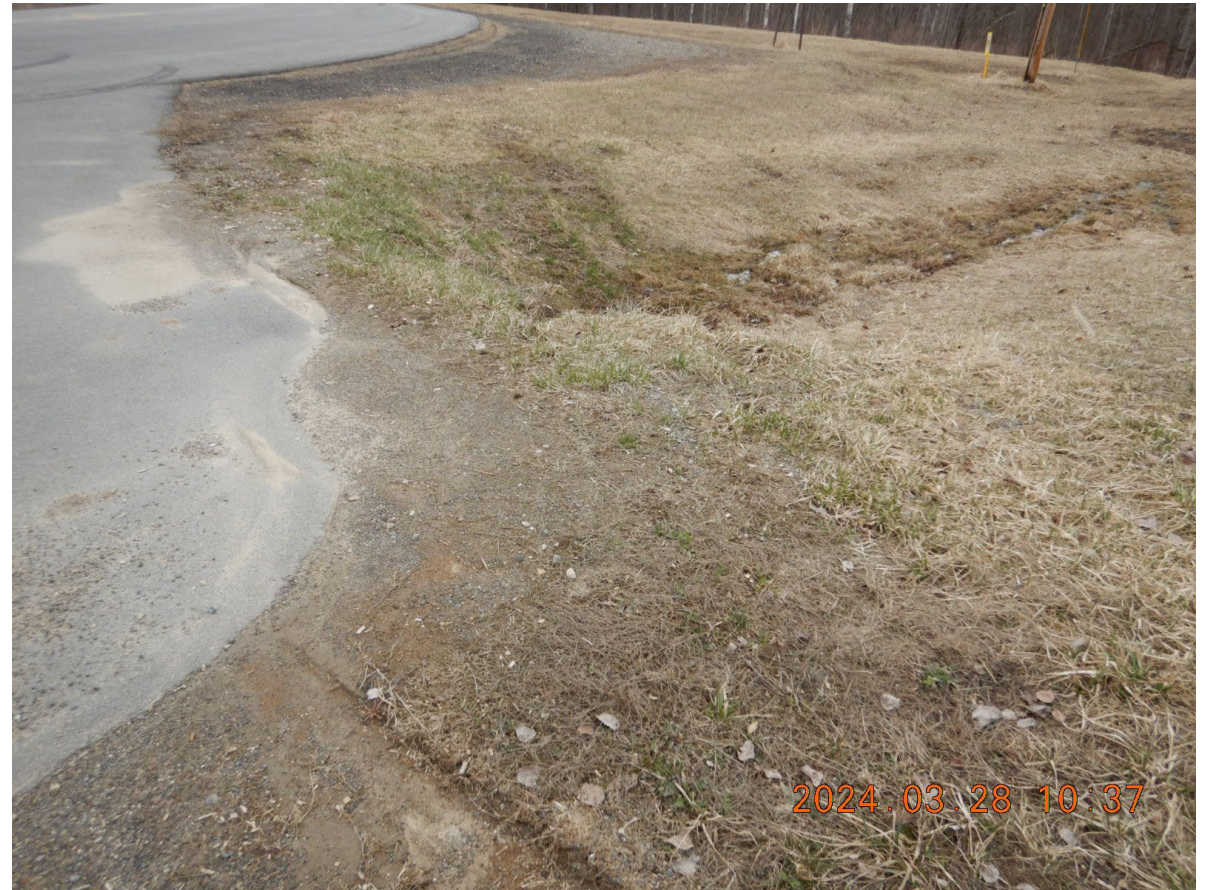
DSCN2729 - Stormwater drainage along Trade Drive – some dirt seen on roadway
