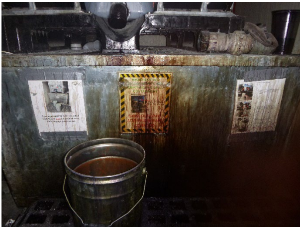
Photograph 10: Daily Tank Area.
