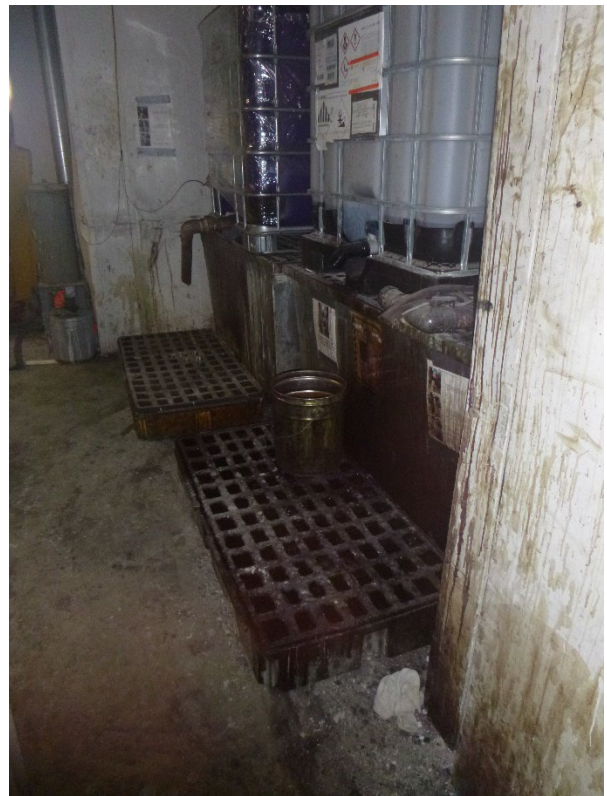
Photograph 12: Daily Tank Area.
