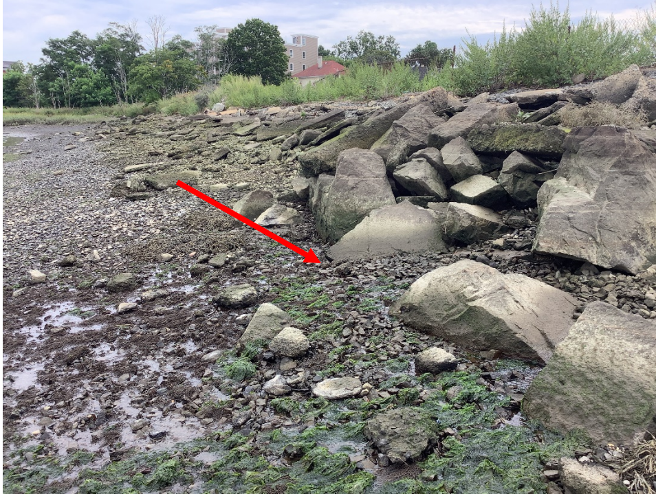
11. Bates: Collapsed outfall on the beach to the north of the baseball field at the end of Bates St. Sample point indicated by a red arrow.
