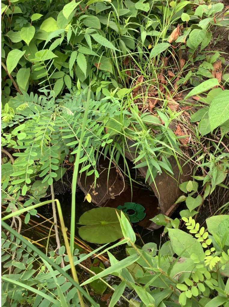
7. 51LV Ave: Outfall on Flax Pond located near 51 Lake View Avenue. Dry at the time of recon inspection. Not visited during sampling inspection.
