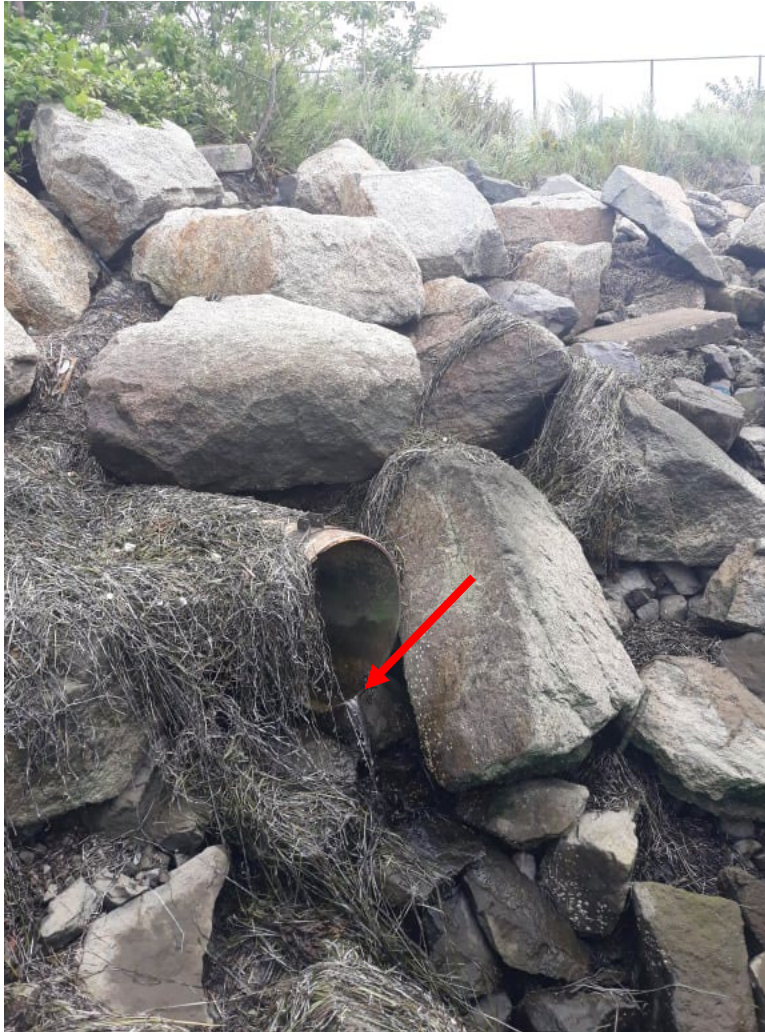
18. Surfside: Outfall located on the southeast side of the Ocean Shores apartment complex. Sample point indicated by a red arrow.
