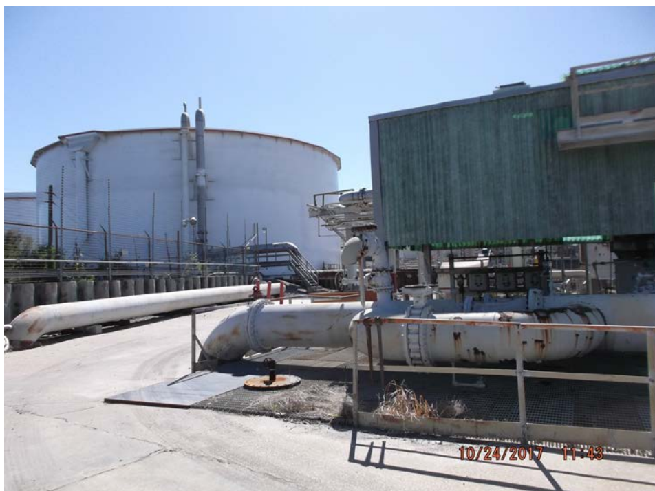
Photo 3 – Piping where alternative sample point can be added for outfall 009. Two of four surge tanks in background.
