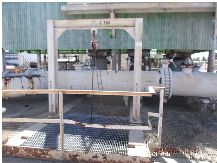
Photo 1 - Sump with Gate Valve to allow emergency overflow at outfall 009. When necessary, gate valve opened manually with pulley. Samples for 009 taken within sump.
