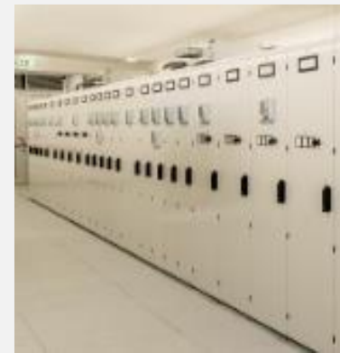
Timeline example and picture: HV/MV substation with SF 6 MV switchgear, South Germany
