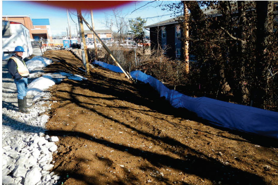
Photo 21, Sediment accumulation against a section on silt fence.
