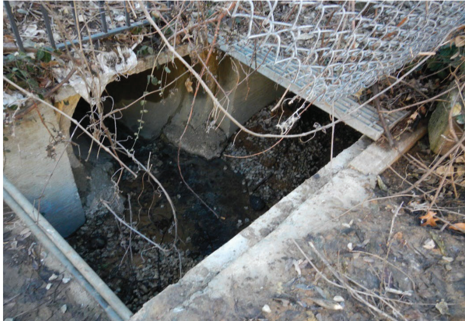
Photo 23, Outfall 01 with no sediment controls.
