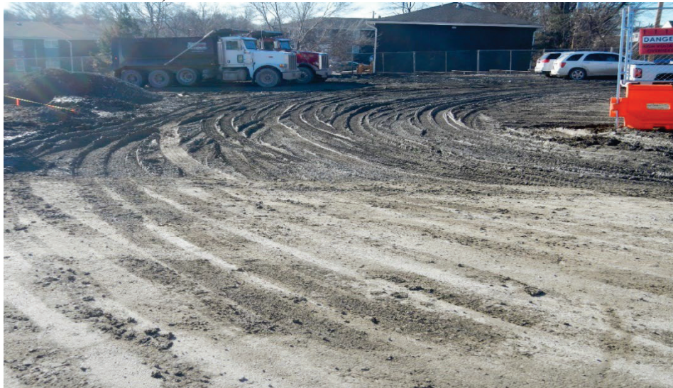
Photo 4, Lack of BMPs at one of the site's entrances.
