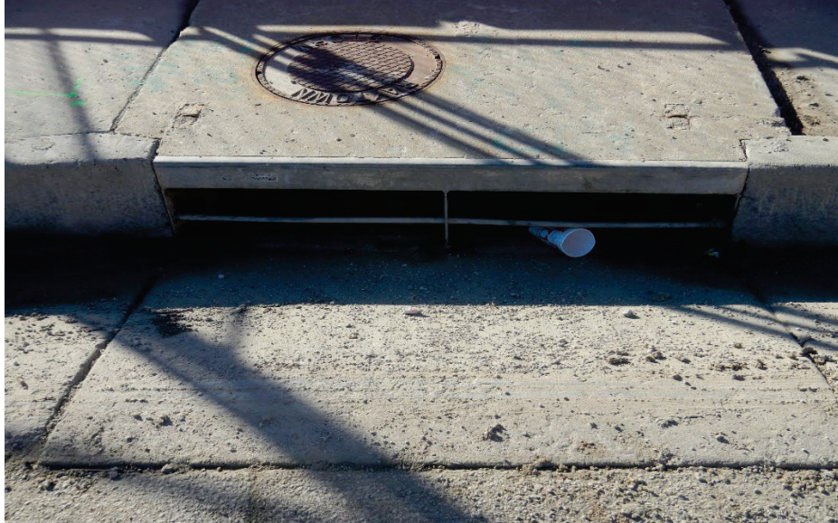
Photo 5, Sediment entering the stormwater inlet curb at 61 st Street.
